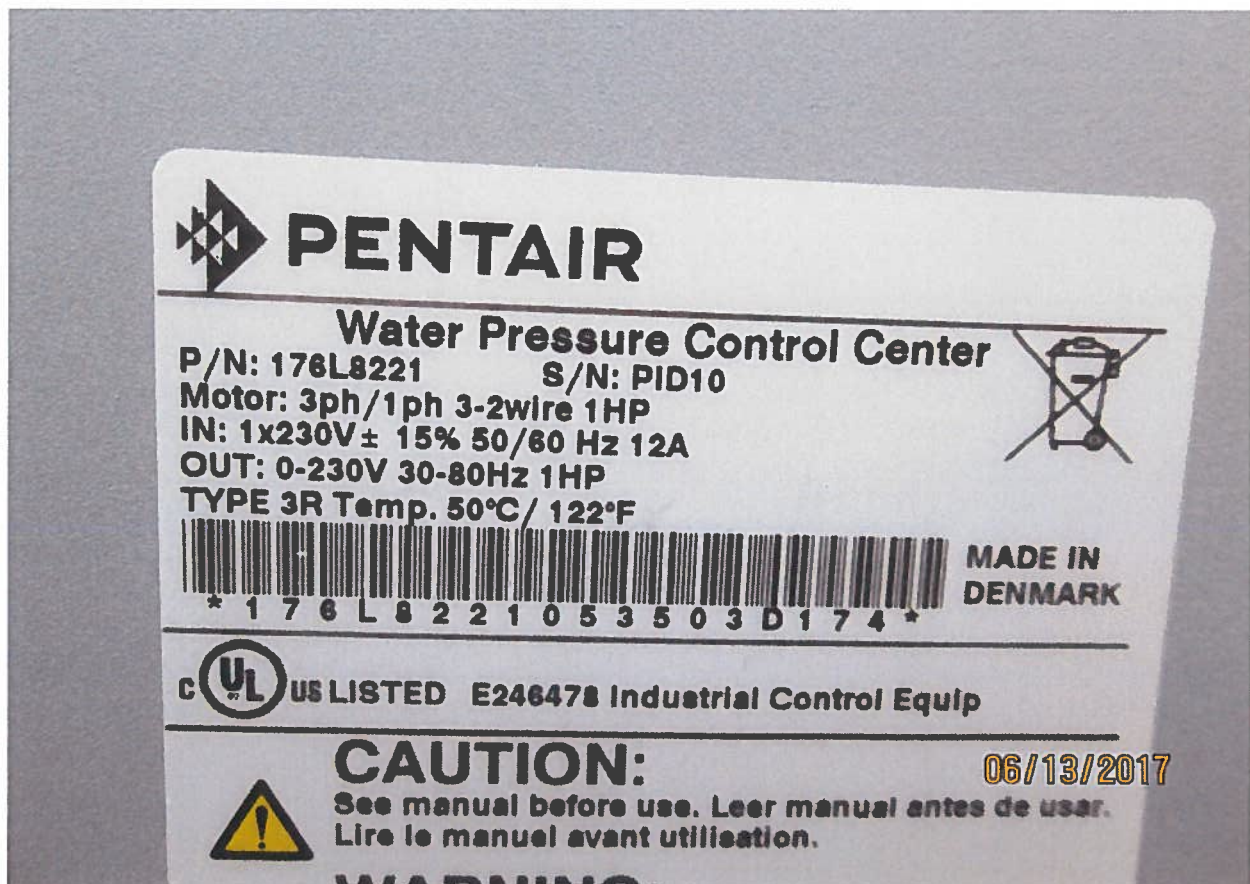
1hp pump in well.
