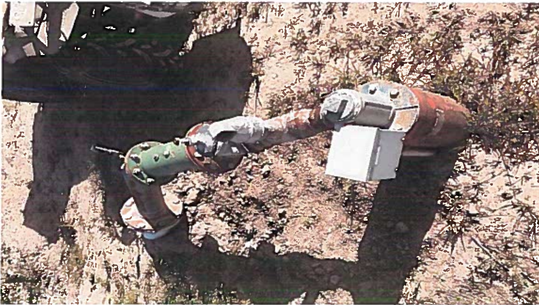
Picture of POD showing 6" discharge pipe heading into ground and towards pivot head.
