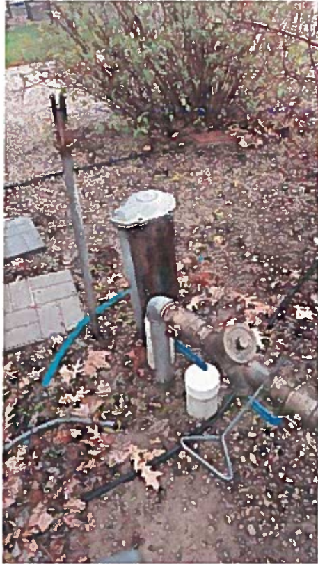
Picture 1: The well head located just north of the house on the Johnson property. The well is 6 inches in diameter. A 5-horsepower pump moves water from the well into a two inch mainline that leads into the sprinkler system
