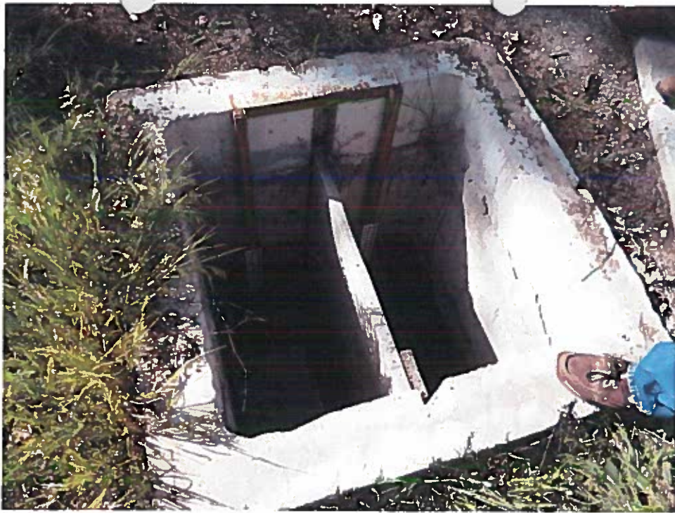
Measuring device control box
