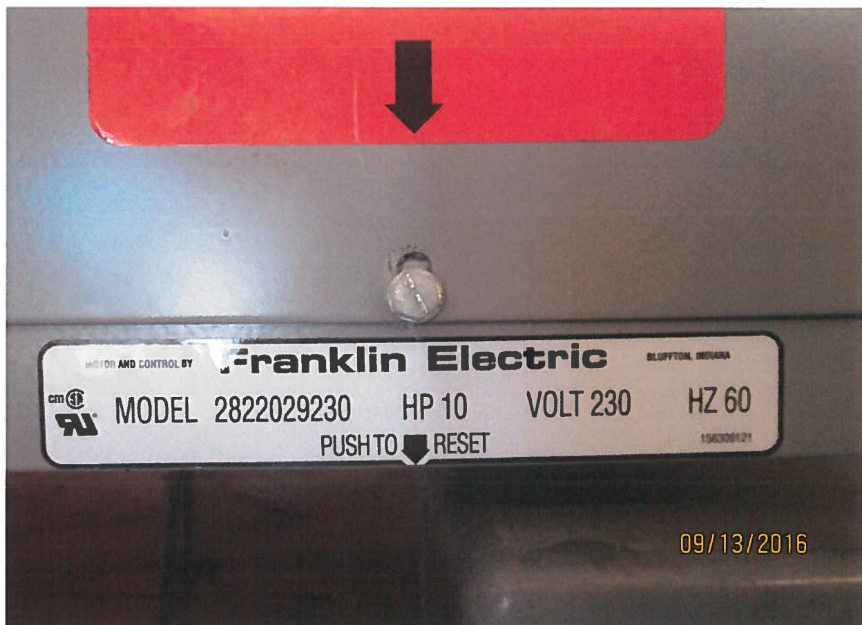
Franklin 10hp pump in well.
