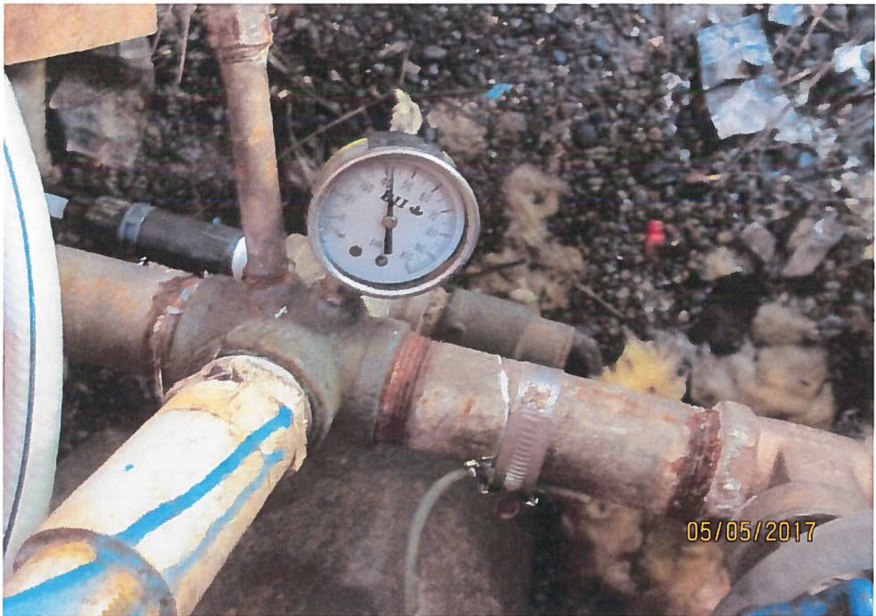
Pressure gage on system reading 42 psi.
