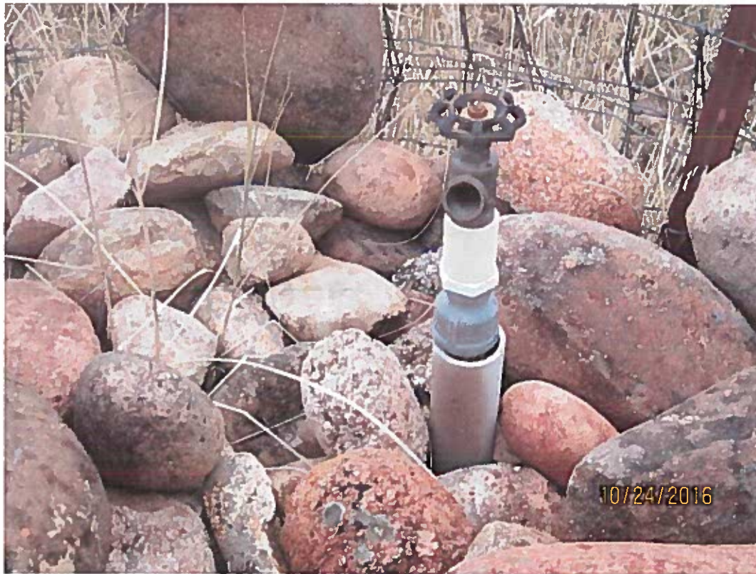
Some risers have a sprinkler, while others have a hose bib valve.
