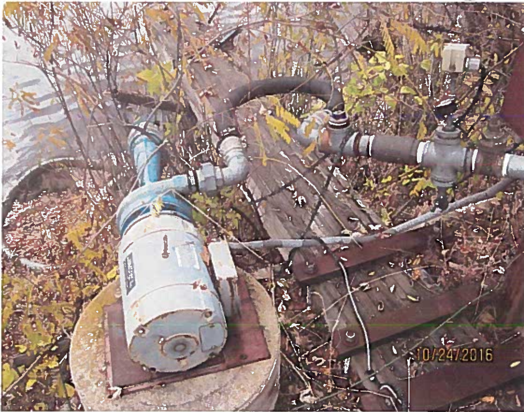
7.5 HP pump that diverts water through a 4" PVC pipe 700' up to the storage pond.
