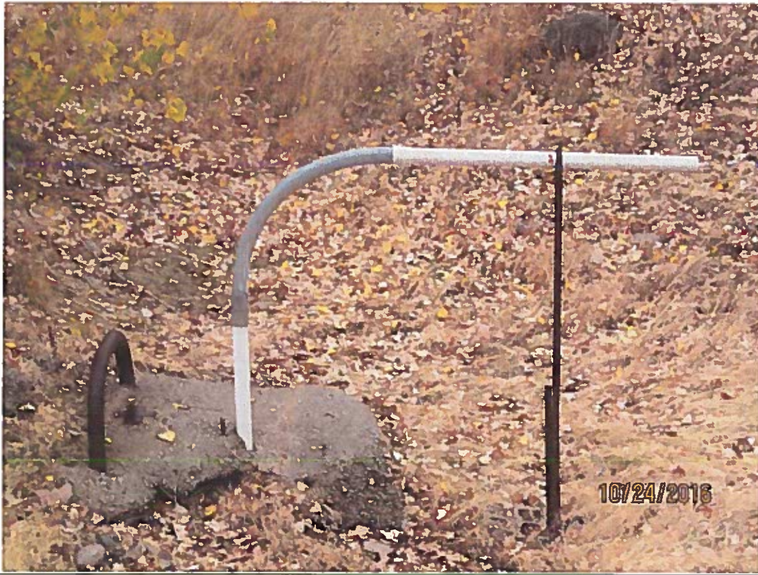
Outlet for the diverted water that fills the storage pond.
