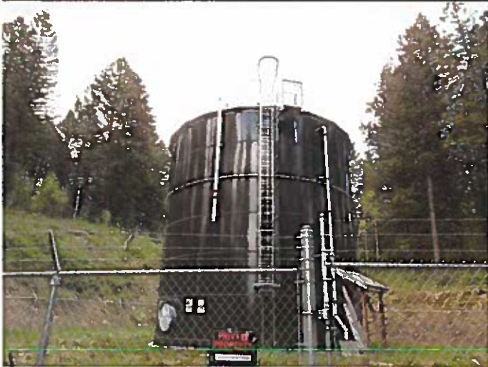
Top Tank 132,000 gallon
