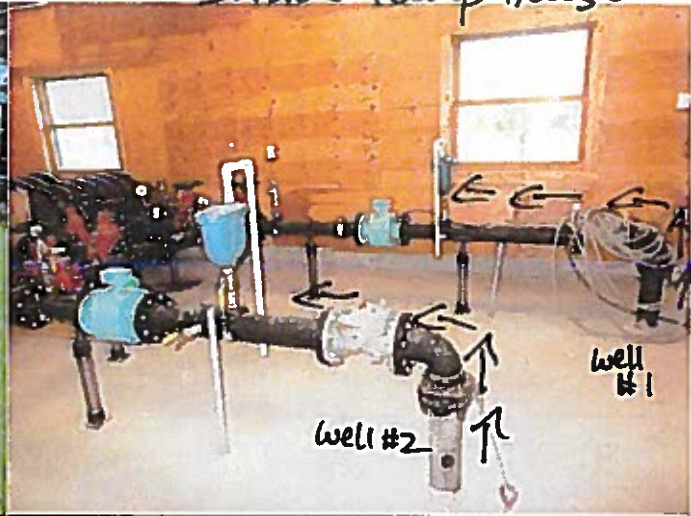
Inside Pump House
