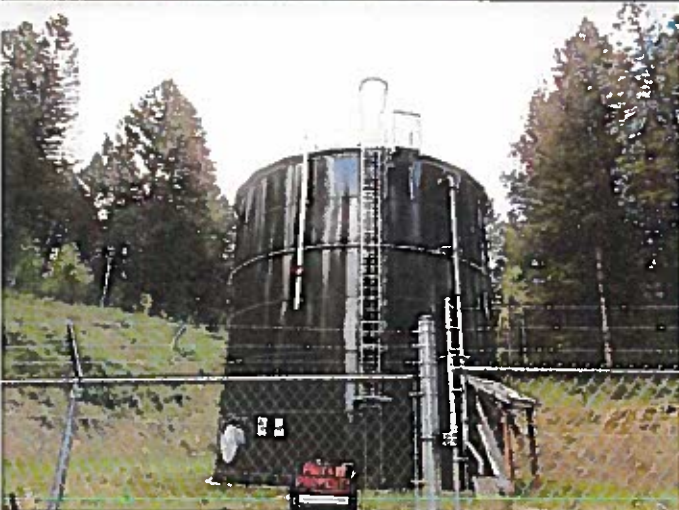
Top Tank 132,000 gallon
