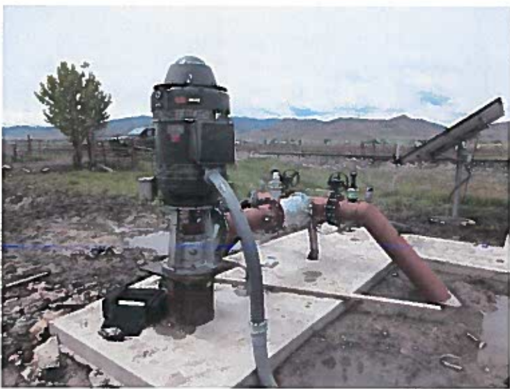
Pump with piping system
