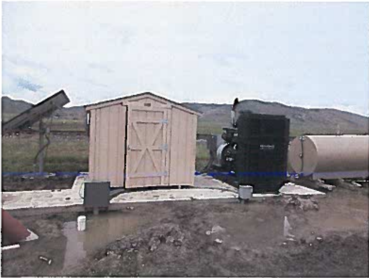
Pump house with Isuzu motor on the right
