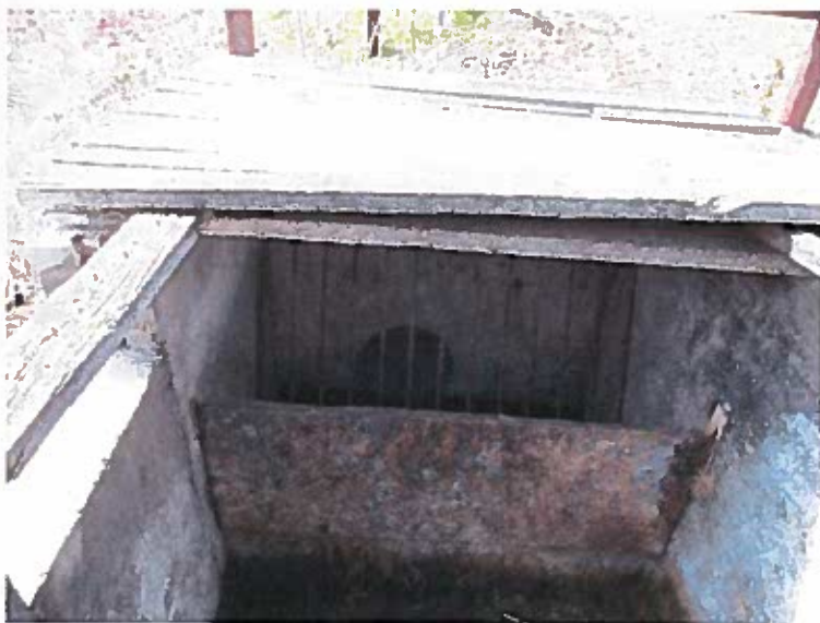
Looking down into the weir at the 12" Plastic Pipe that carries water down to the irrigation system and Ponds.
