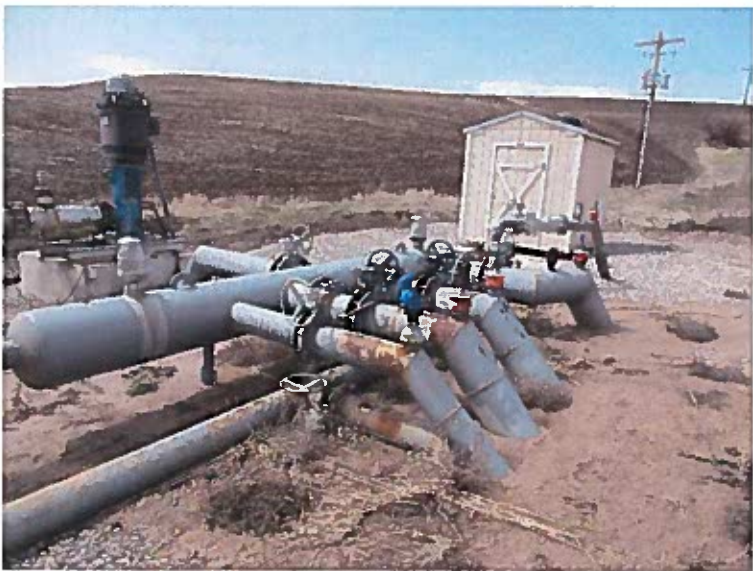
Close up of system. Pump is not hooked to this system.
