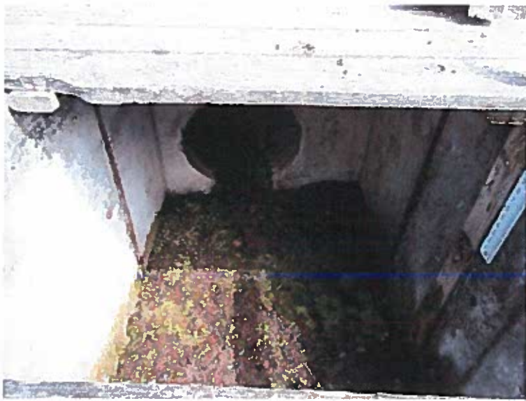
12" CMP that brings water from the springs in the hills to the weir.
