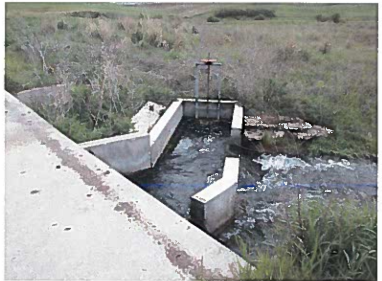
Structure to divert water through headgate
