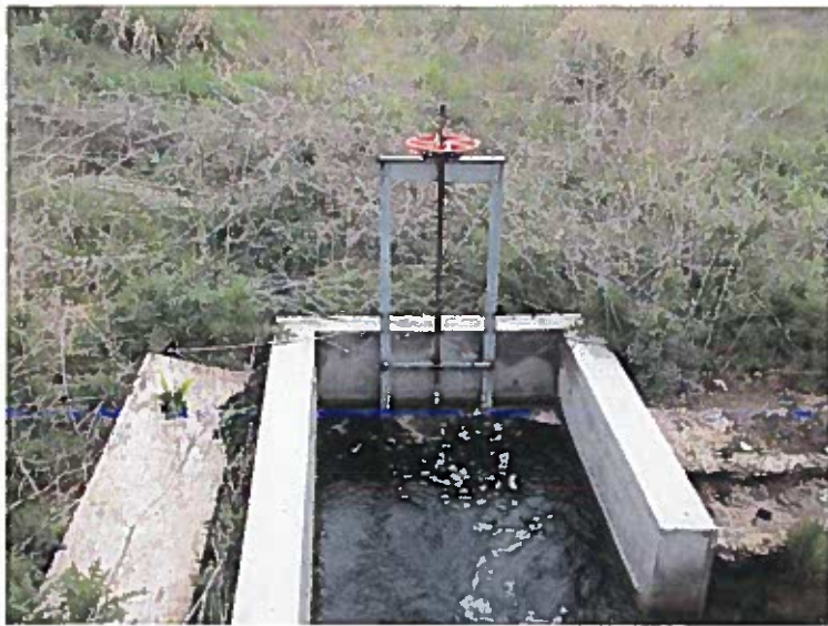
Point of Diversion headgate into 12" CMP
