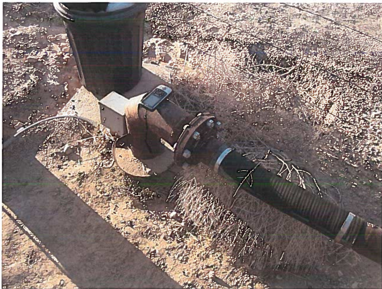
Figure 3 Another view of the well head as it comes out of the ground.
