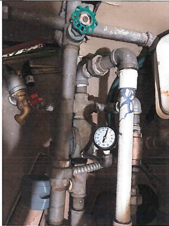
Photo 2. The pressure gage in the photo is located in the garage of the house. With one big gun running the pressure was at 62 psi.
