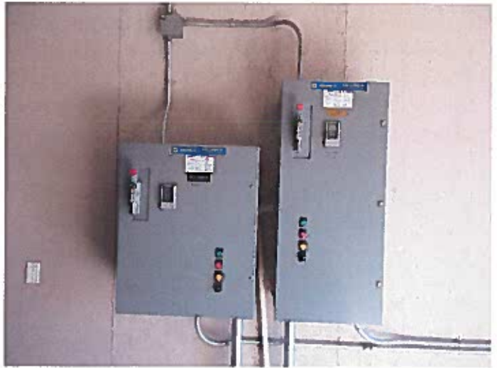
Electrical system for pumps
