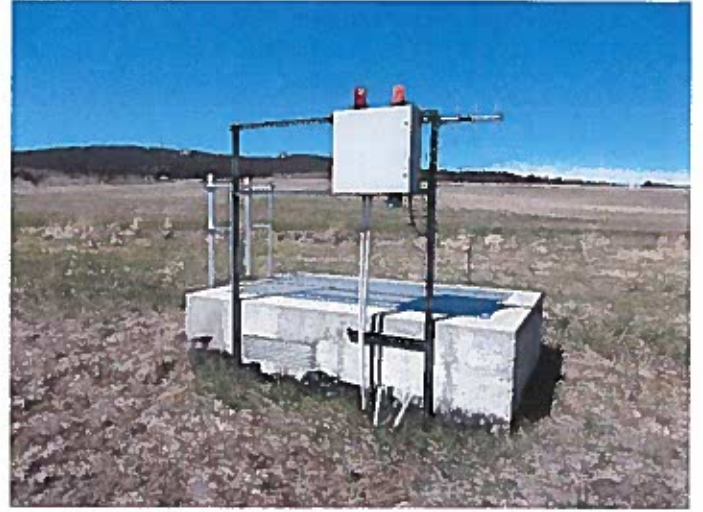
200,000 gal storage tank access point
