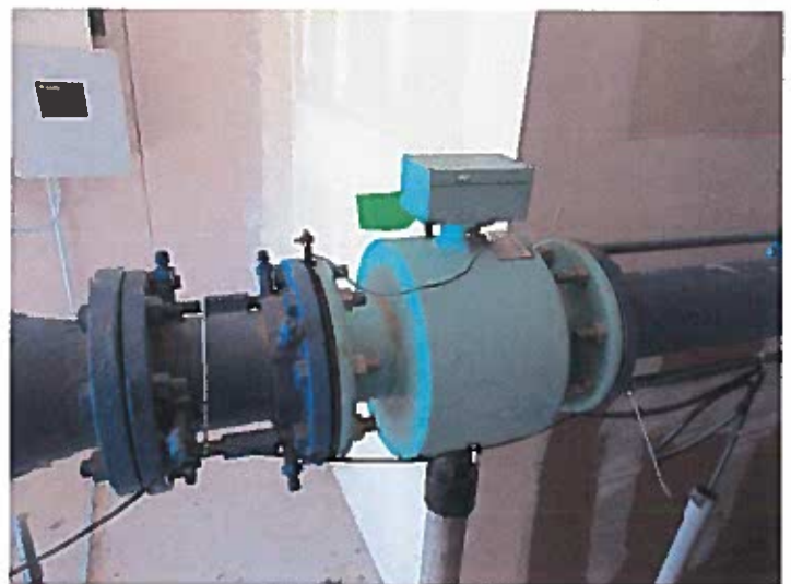
Mag Flow meter installed
