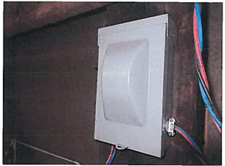
Electrical box closed with tab that can be locked by Watermaster if need be.
