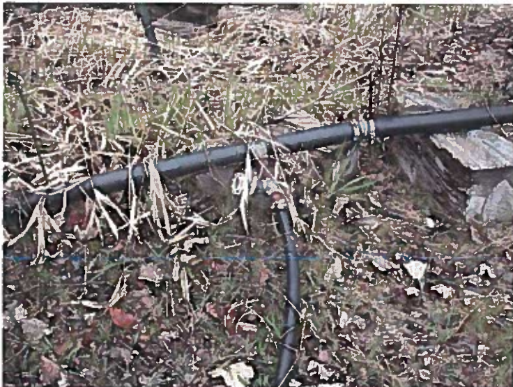
T off main 2" PVC lin that runs to the east. This is used to hook up a hose and a rain bird.
