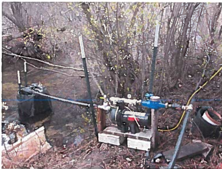
Pump hooked up to power supply and to pipe pulling Water from Freeman Creek
