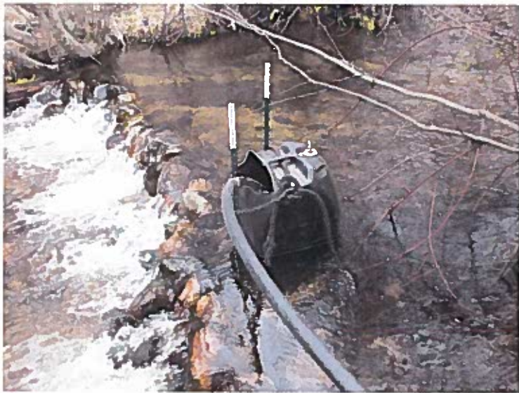
2" PVC pipe running to stream with 55 gallon plastic barrel protecting the piping and keeping debris out.
