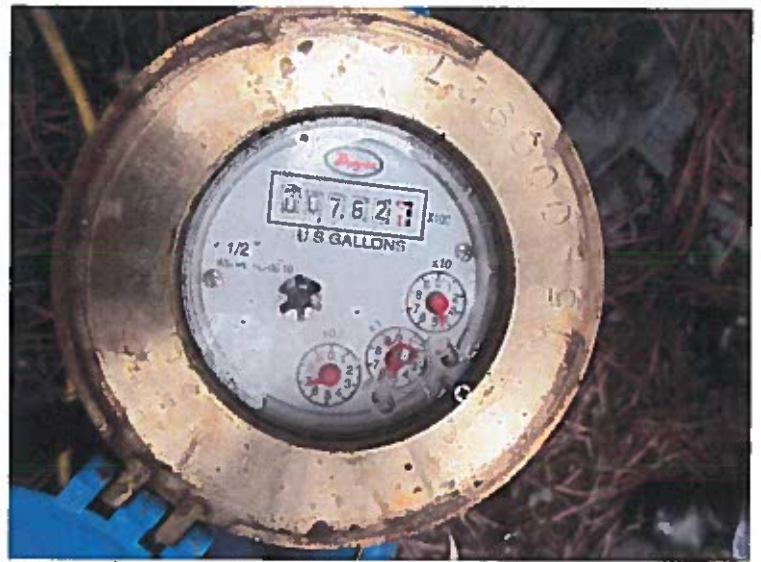
Dwyer flowmeter installed on pump. x100 multiplier
