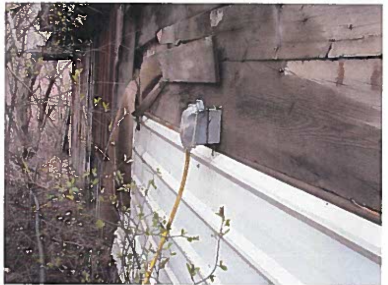
Electrical box inside it linked to this outlet that pump can then be hooked up to for power
