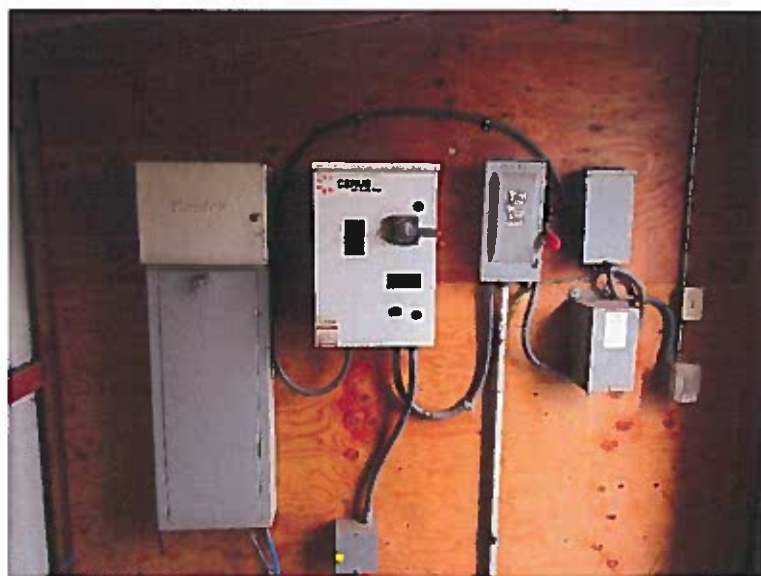
Whole electrical system
