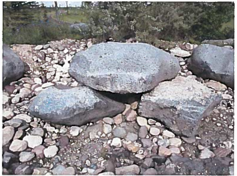
Pipe under this big rock is where water is diverted to the pond
