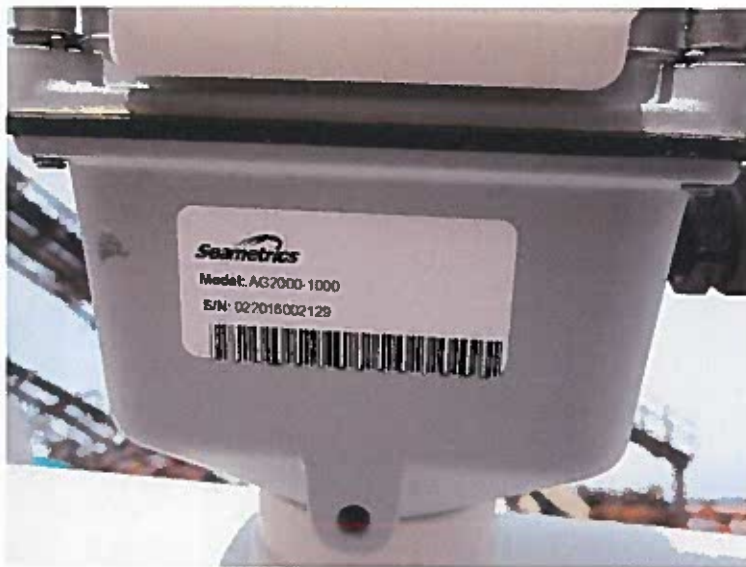
Serial number and model of installed flow meter.
