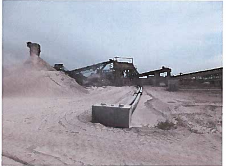
Pipes rung from washing station to discharge Site.
