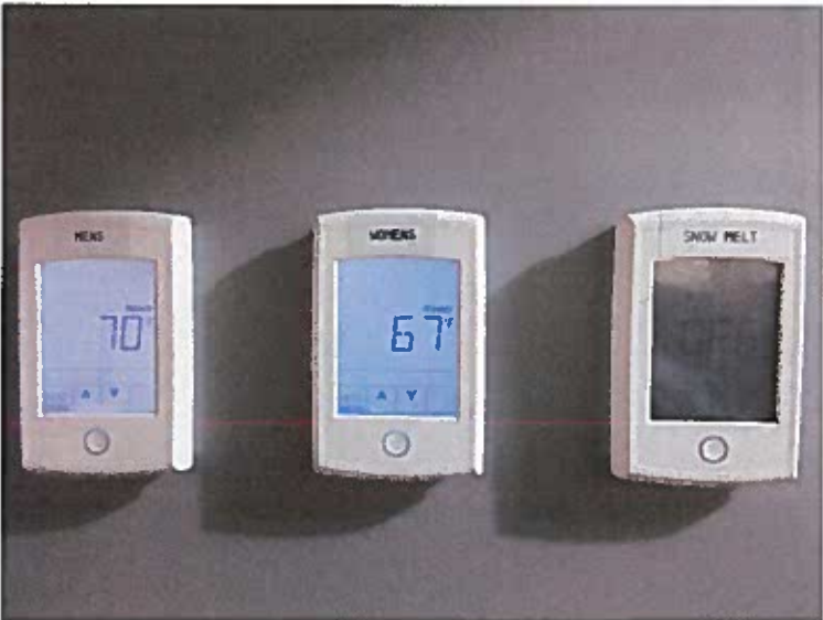
Thermostats for heated floors and sidewalk
