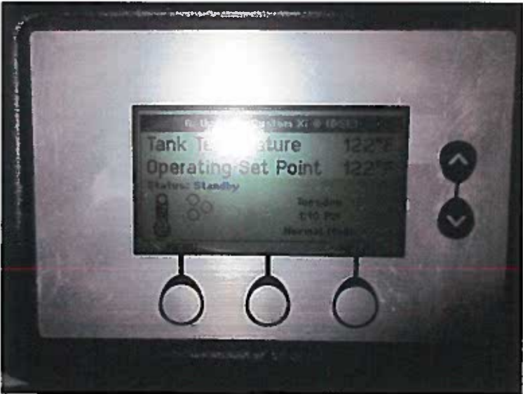
Temp gauge on hot water holding tank
