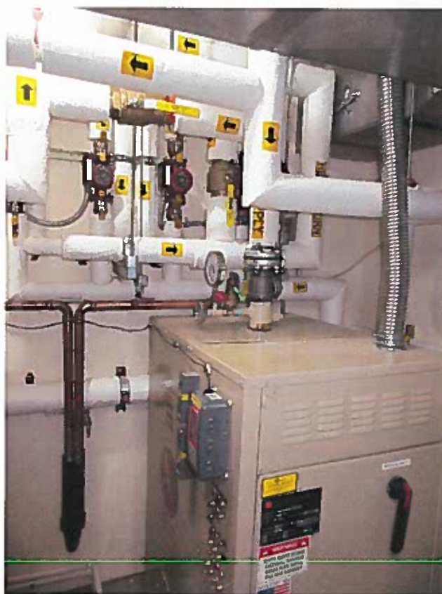
Water going into boiler #1
