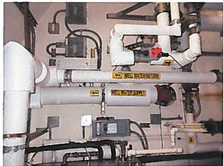
Start of system. Well water comes out of wall into a red elbow and is measured by a ABB flow meter above it.
