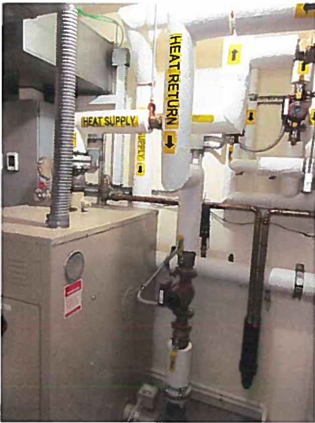
Boiler #2 on the left and return flow to injection well. Red flowmeter can be seen in the middle of pipe.
