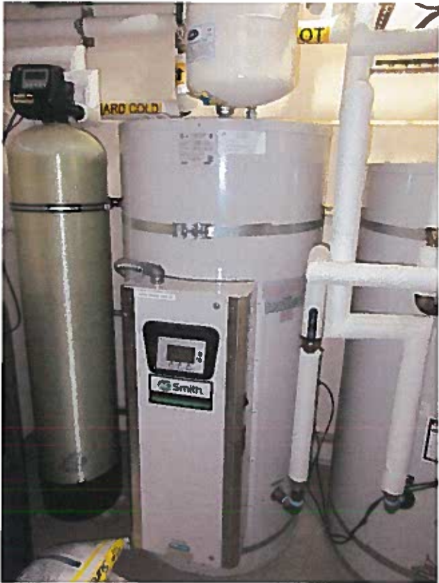
Hot water holding tank
