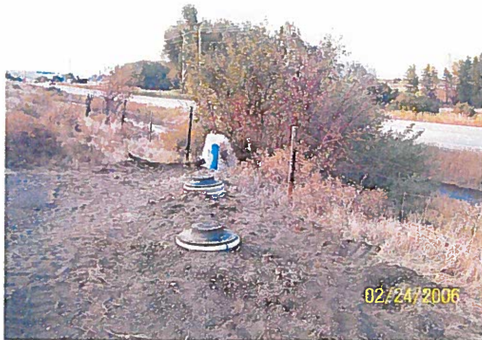
Terminus of the Sam's Hollow mitigation pipeline.
