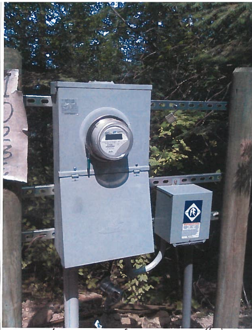
Meter Box is Locked
