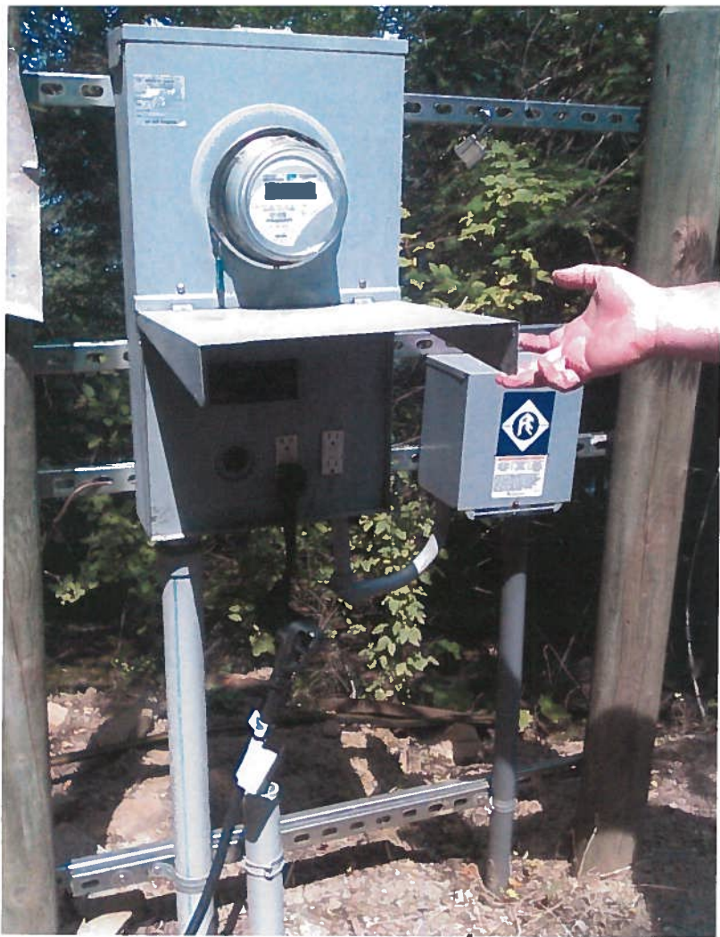
Meter Box with RV hook up
