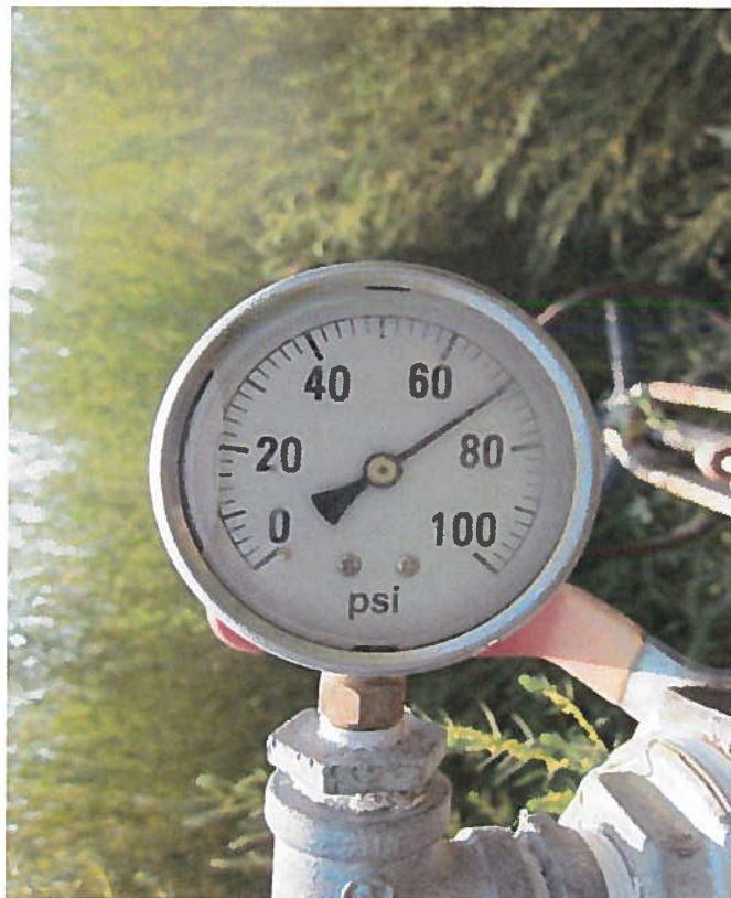
Figure 4: Pressure gauge on well head
