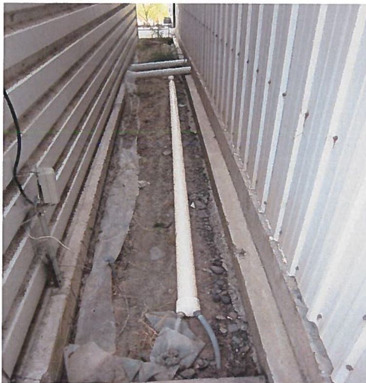
Figure 2: Pipes for heating system between the house and shop
