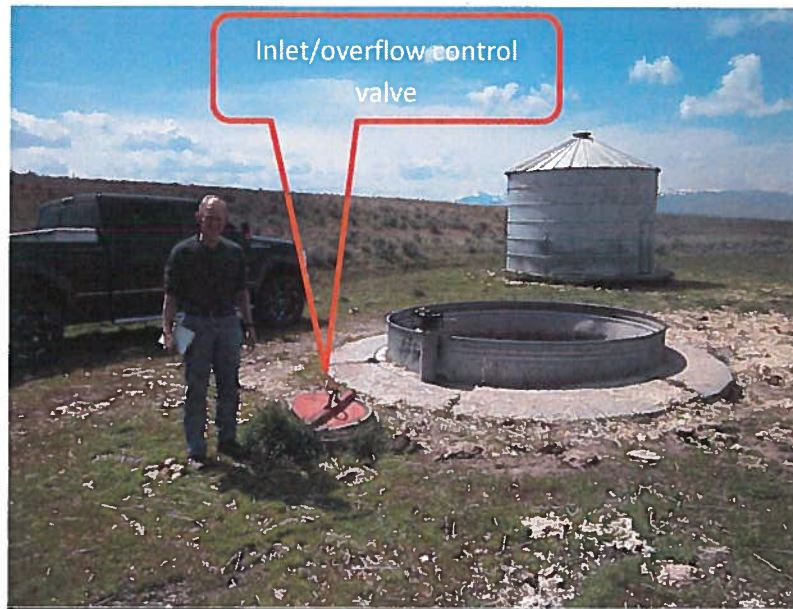
Figure 1: 12S28E15NENW . Elevation 4972 ft. (west of unnamed spring). First trough fed by spring with sub-surface inlet control valve/overflow control valve.
