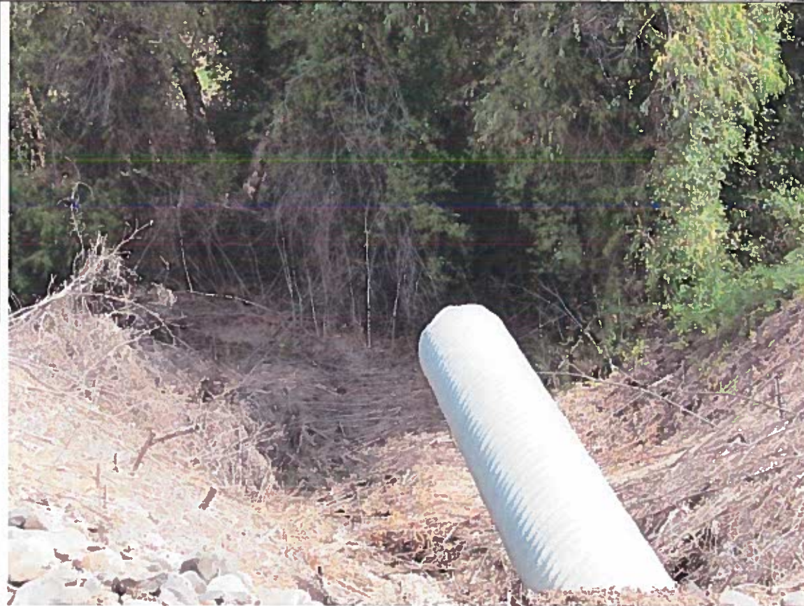
Discharge pipe across the road from the 27 acre parcel. Water can be returned to the stream or be diverted to the drain east of the 27 acre parcel.
