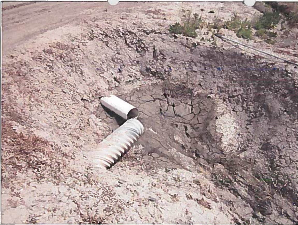
Catch basin at the end of the ditch. The location is shown on the system diagram as drain 1.
