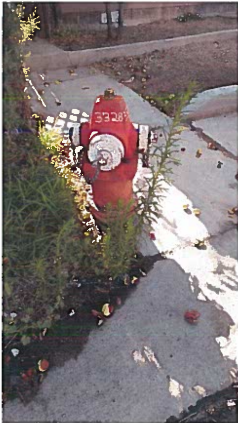
Figure 6 The hydrant located in the southeast of the subdivision.
