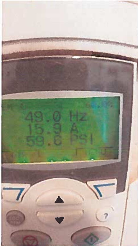
Figure 3 A digital readout screen on the pump control box showing the pressure at the pump at ~60 psi.
