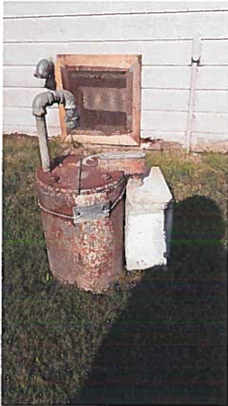
Figure 1 The well located in Lot 2 Block 1 of the Greenleaf Subdivision. The tag shown is the IDEQ water quality tag, not the well tag.
