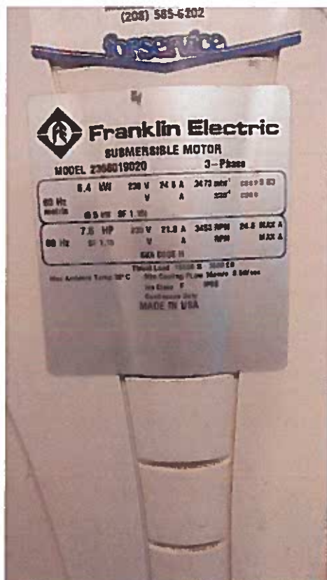
Figure 2 The specifications for the submersible motor showing that the pump is 7.5 hp.
