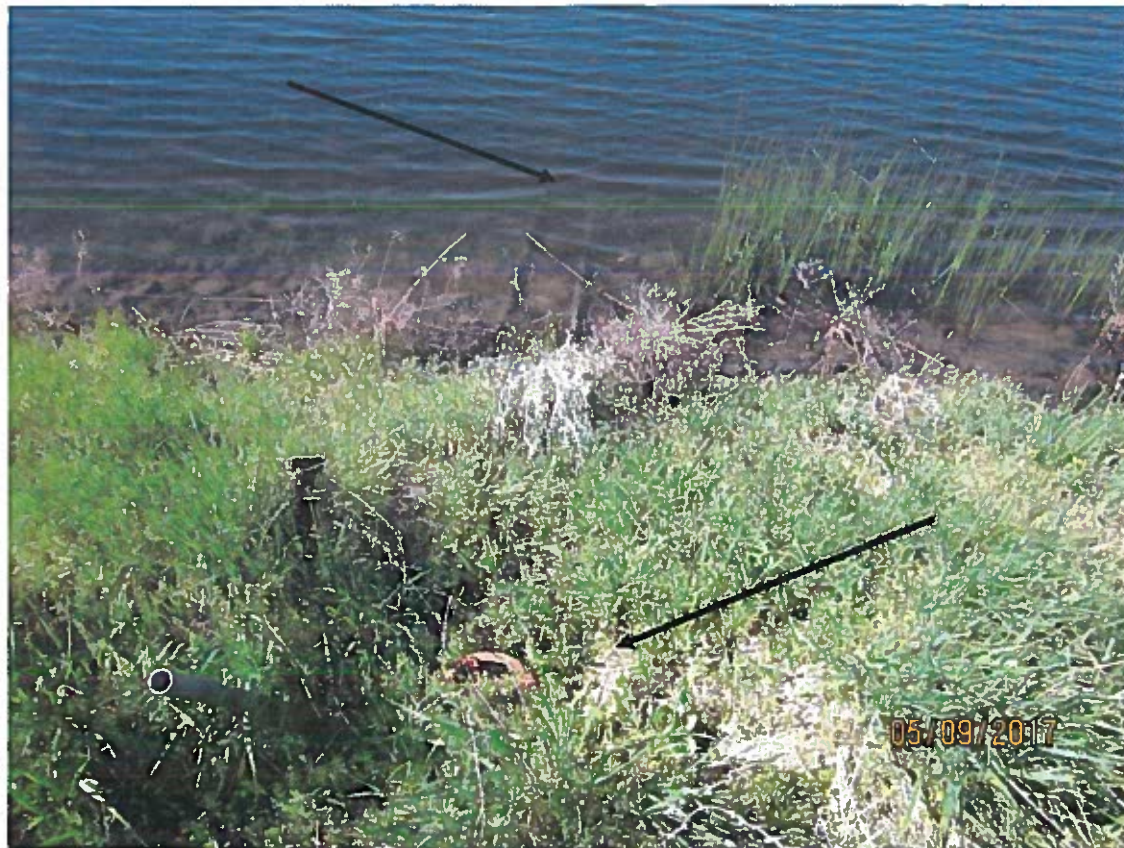
Gate valve that allows water to flow to the toe of the dam dike. The valve is 15' deep. The 15' depth was used as the maximum depth of the reservoir.
