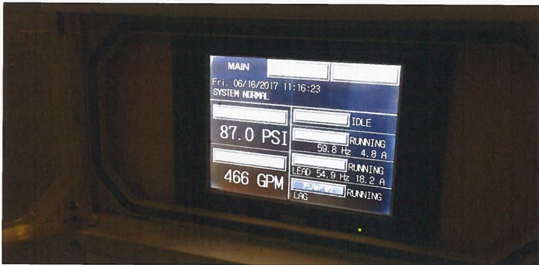
Motor control display for park pumps. Note that one 30-hp pump (Pump # 2) is operating at 54.9 hz (less than 60 hz, full speed) and second 30-hp pump (Pump #1) is idle. The 5-hp pump is running at full capacity.
