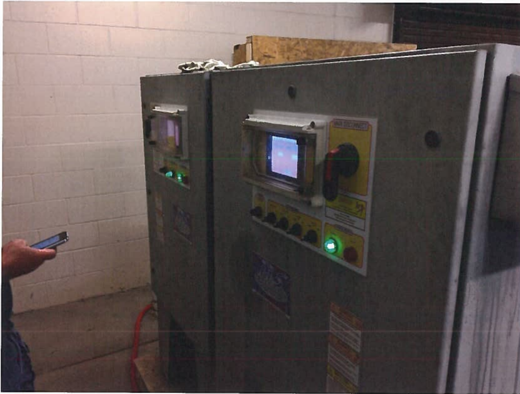
Motor control panels. Panel on right encloses controls for Park pumps (two 30-hp vertical turbine and one 5-hp submersible). Panel on left encloses control for Barber Station pump (63-34258).
