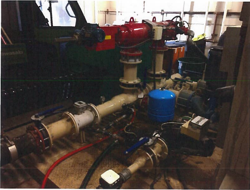
Pump house plumbing. Park irrigation piping in background with red automatic filter, beige mag meter, and blue handle butterfly valve. Barber Station (63-34258) irrigation piping in foreground with black automatic filter, blue butterfly valve, and white top flow meter. Motor controls out of picture on right.
