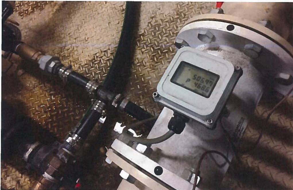
6-inch AG2000 flow meter for measuring irrigation flow through Park pressure irrigation system
