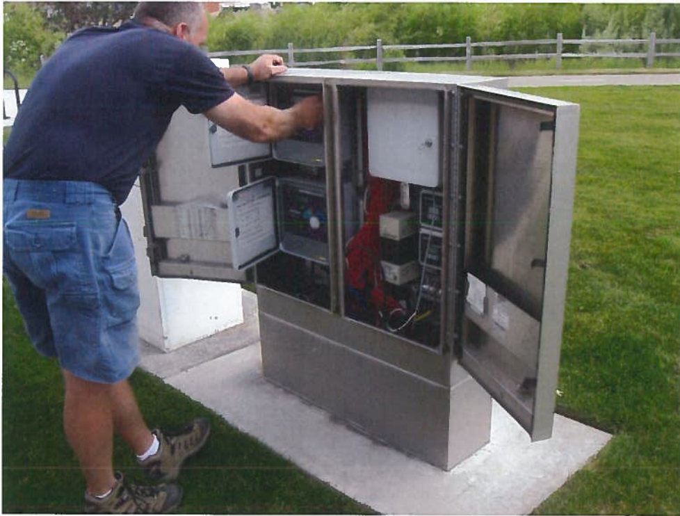
Sprinkler system controls
