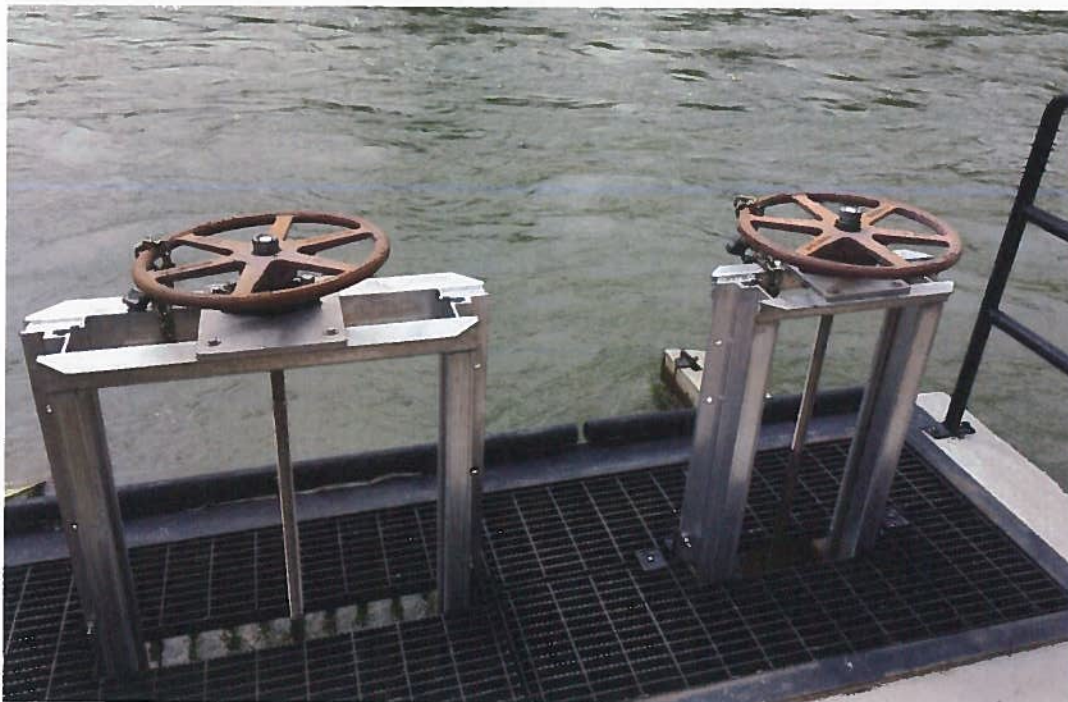
Boise River diversion headgate controls to settling pond; note chains for lockable control.
