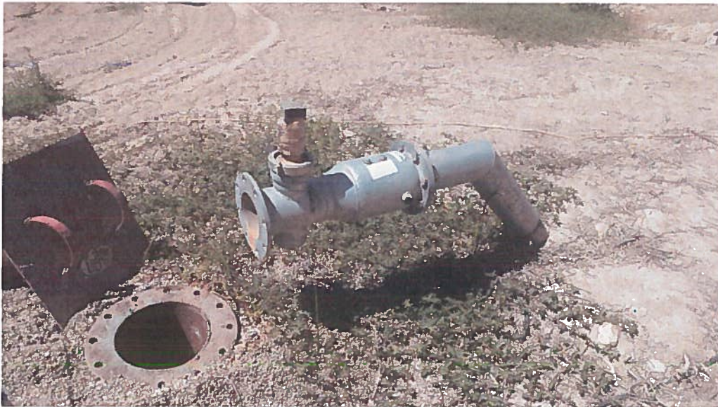
Figure 1 The 12" well used as the POD. According to the farm owner, the well has failed and will be replaced. There was no pump at the time of the exam.
