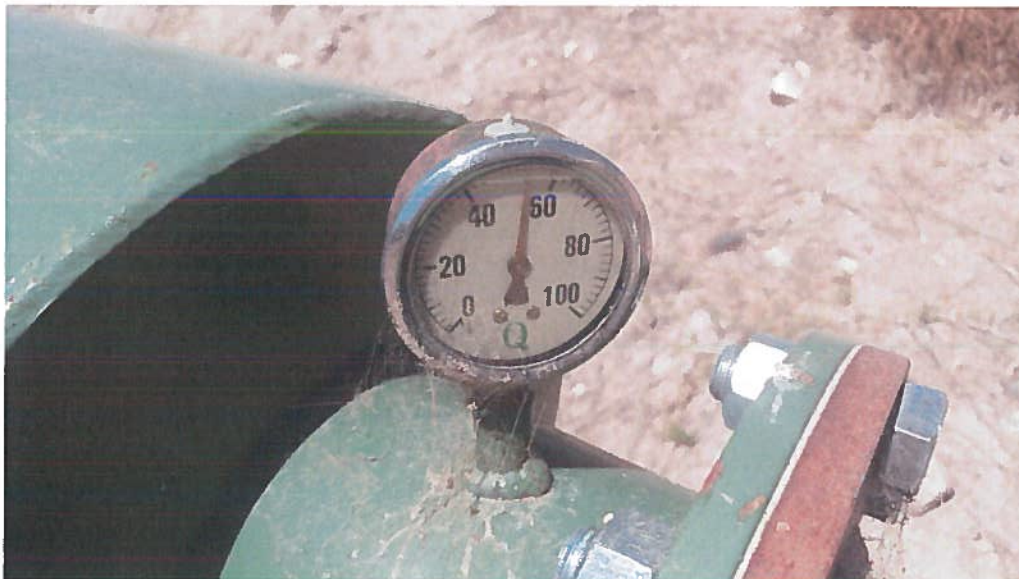
Figure 2 The gage pressure reading at the start of the mainline showing 55 psi. The pressure shown is the pressure when water from the ditch is used.
