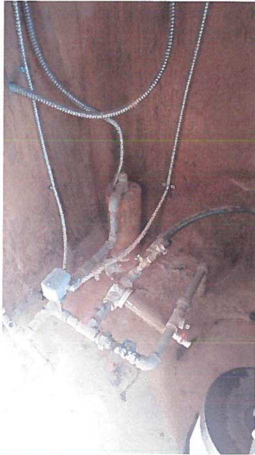
Figure 2 A view of the well head inside the pumphouse which is located directly south of the shop along Gekeler Rd.
