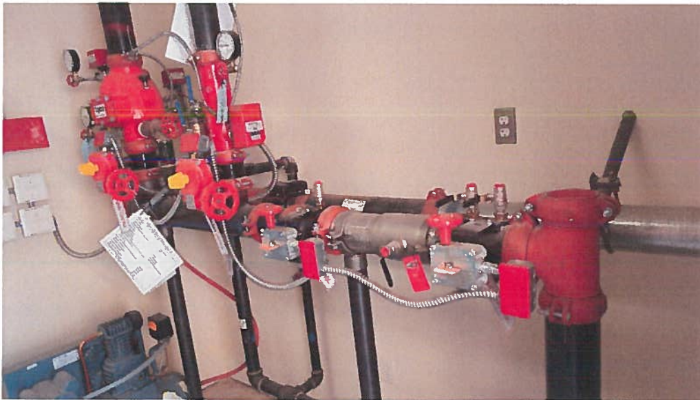
Figure 2 The internal sprinkler system as it comes into the south side of the building from the 8" mainline outside.
