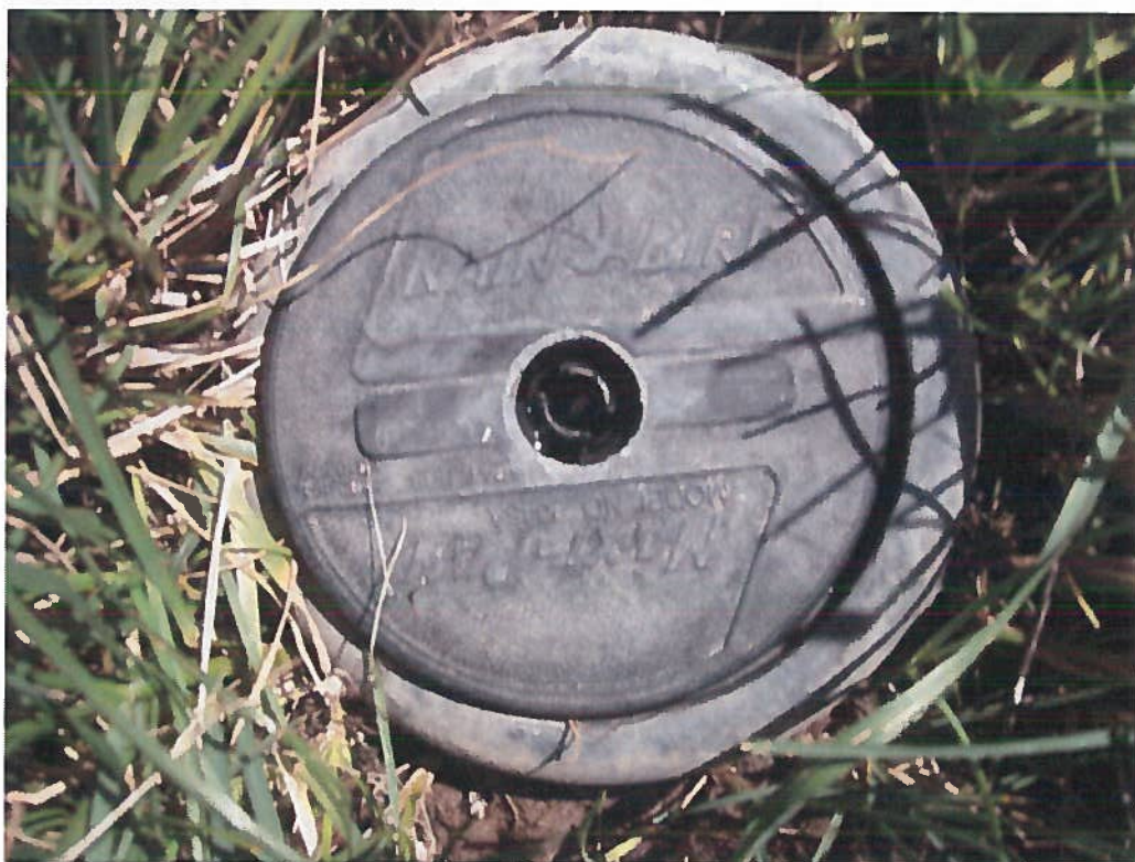
Figure 2 Rain Bird pop-up sprinklers used to irrigate lawn and landscaping.
