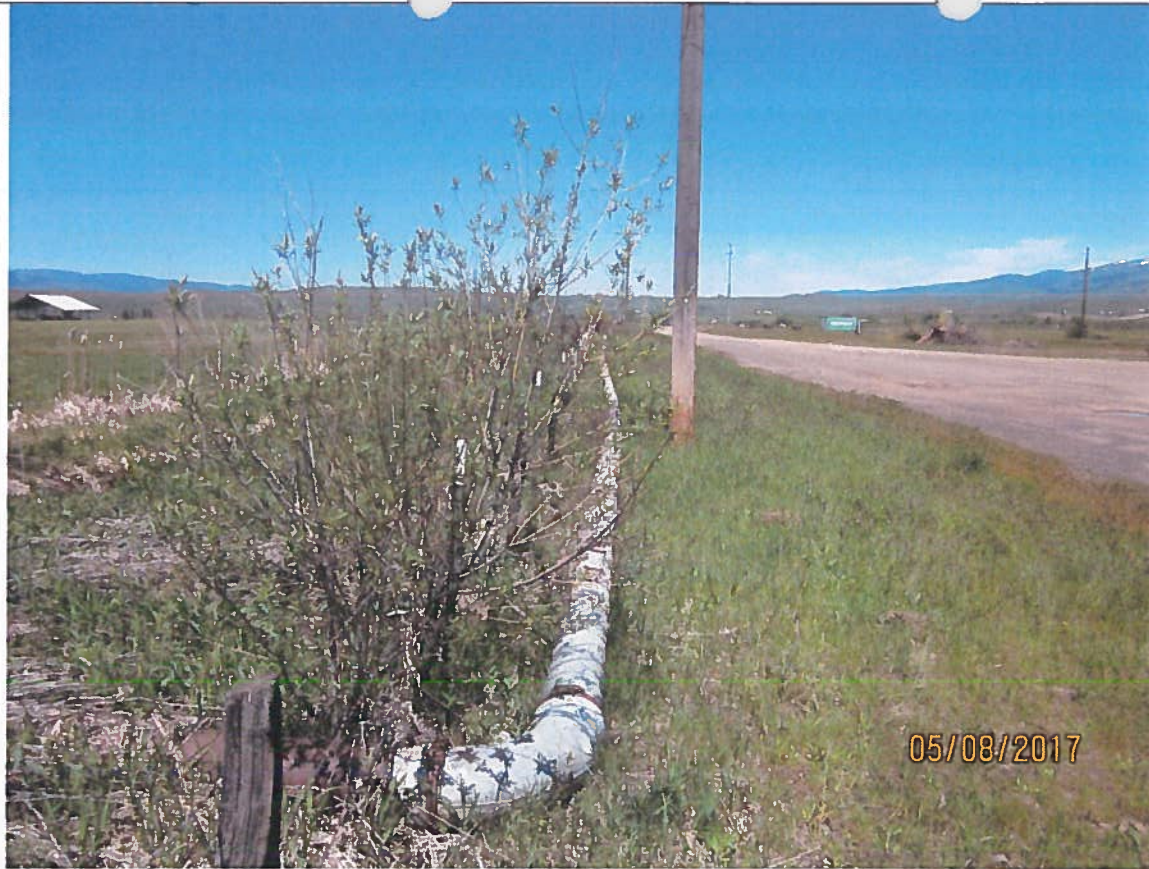
10" aluminum pipe running parallel with Indian Valley Road that carries the water to the ditch along Gray's Creek Road.
