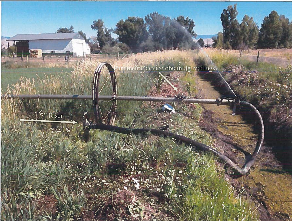
Wheel Line 2 that portrays the connection to the 3" riser. Flow rate at this location was 0.22 cfs for 18 sprinklers.
