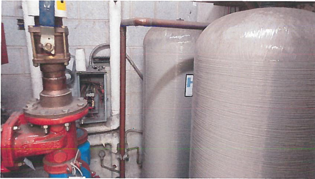
Figure 3 The storage tanks and control box for the well located just inside the warehouse near the well.
