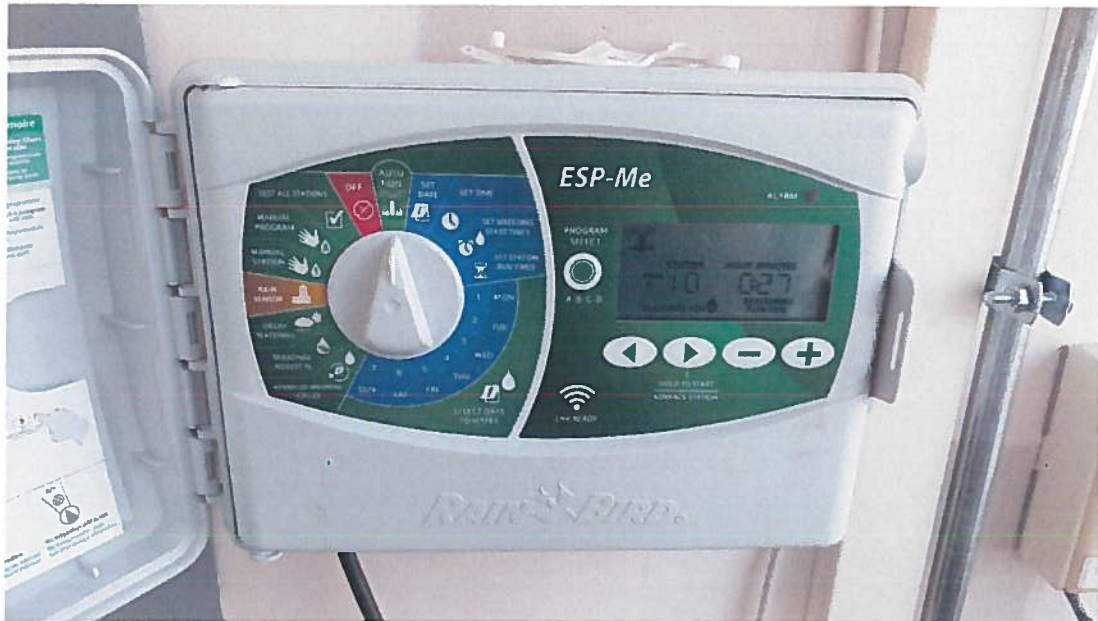
Figure 5 The Rain Bird irrigation control box located in the guard station at the entrance to the warehouse.
