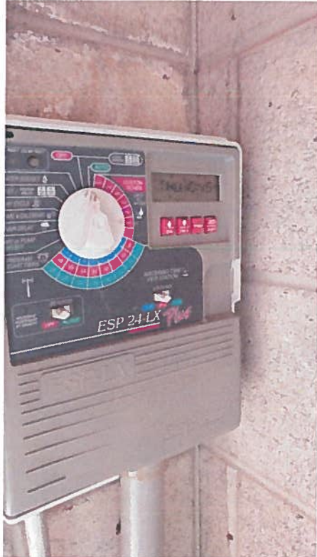
Figure 4 The irrigation box which controls the timing of watering of 20 separate zones of pop up and gear drive sprinklers
