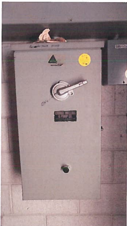
Figure 2 The power control box that sends power to the pump to divert water from the well.
