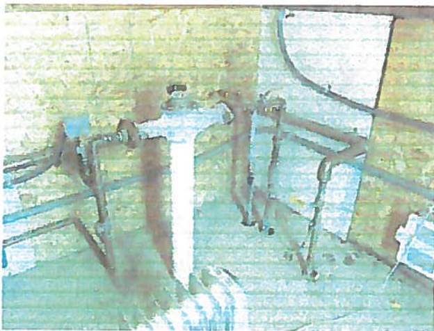
Photograph 9: Well discharge lines
