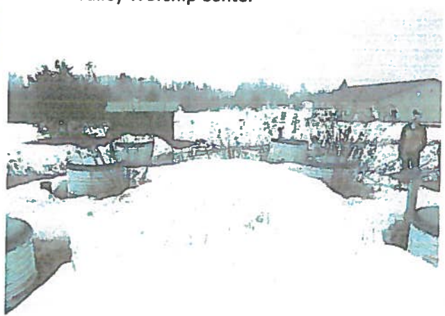
Photograph 18: Storage tank risers and vents
