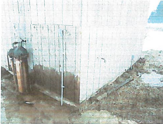
Photograph 17: Flow to waste discharge
