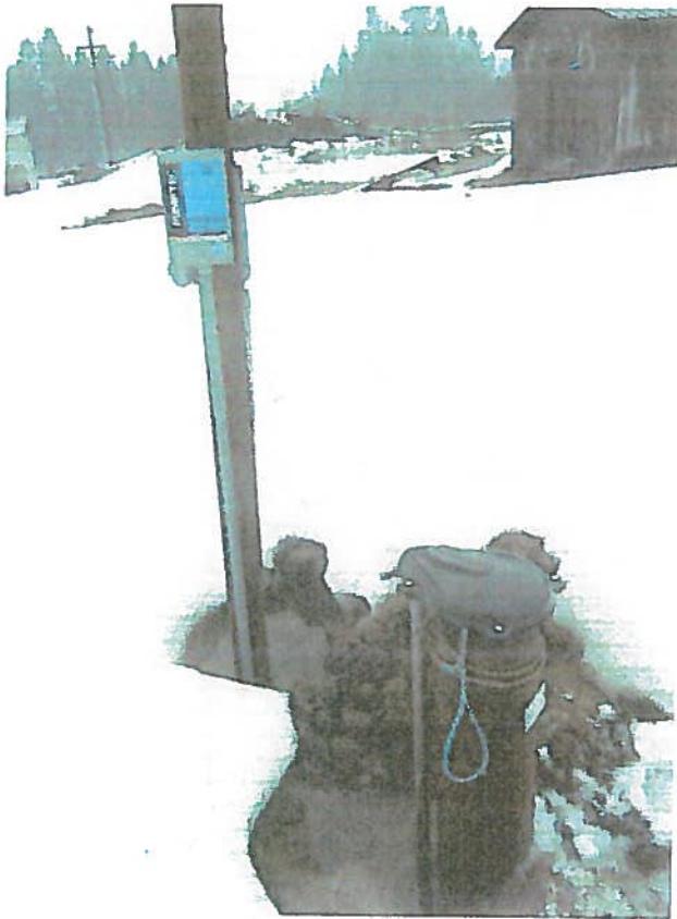
Photograph 3: Well #2 with pump control box
