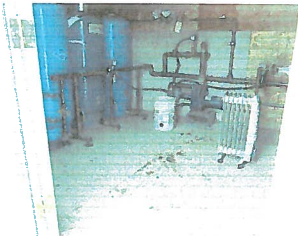
Photograph 7: Inside pump house
