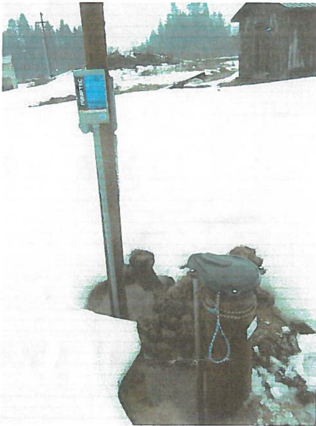
Photograph 3: Well #2 with pump control box
