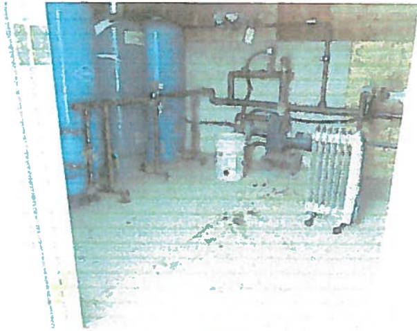
Photograph 7: Inside pump house
