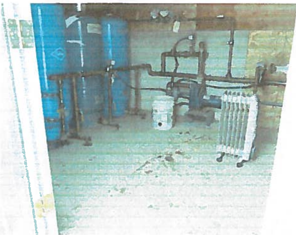
Photograph 7: Inside pump house
