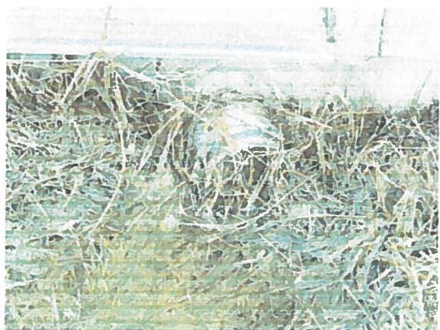
Photograph 16: Pump house floor drain discharge
