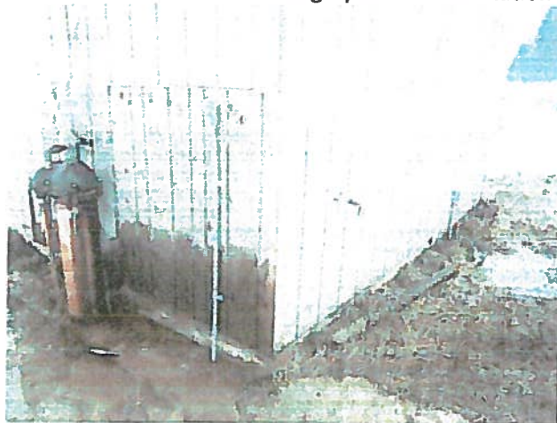
Photograph 17: Flow to waste discharge
