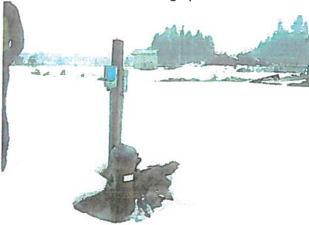
Photograph 5: Well #2 looking toward pump house
