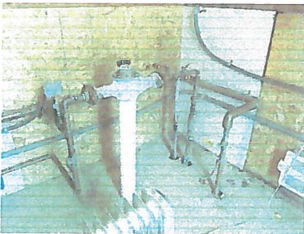
Photograph 9: Well discharge lines
