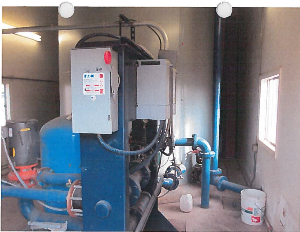
Plumbing inside pump house
