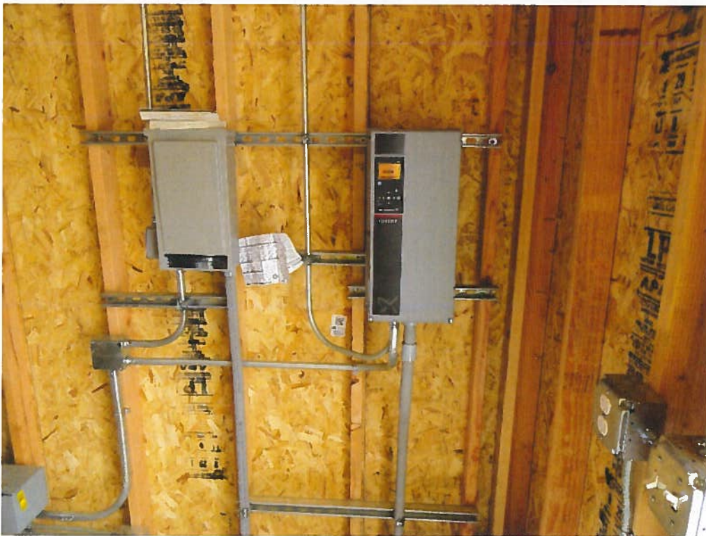
Well pump VFD
