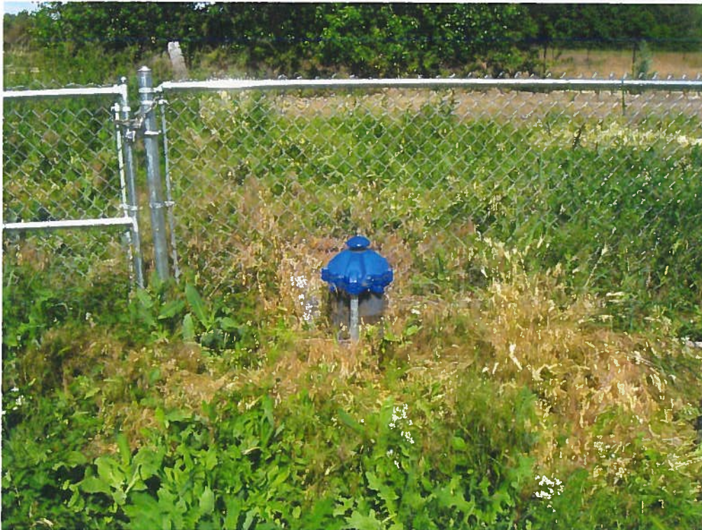
Surface water wet well
