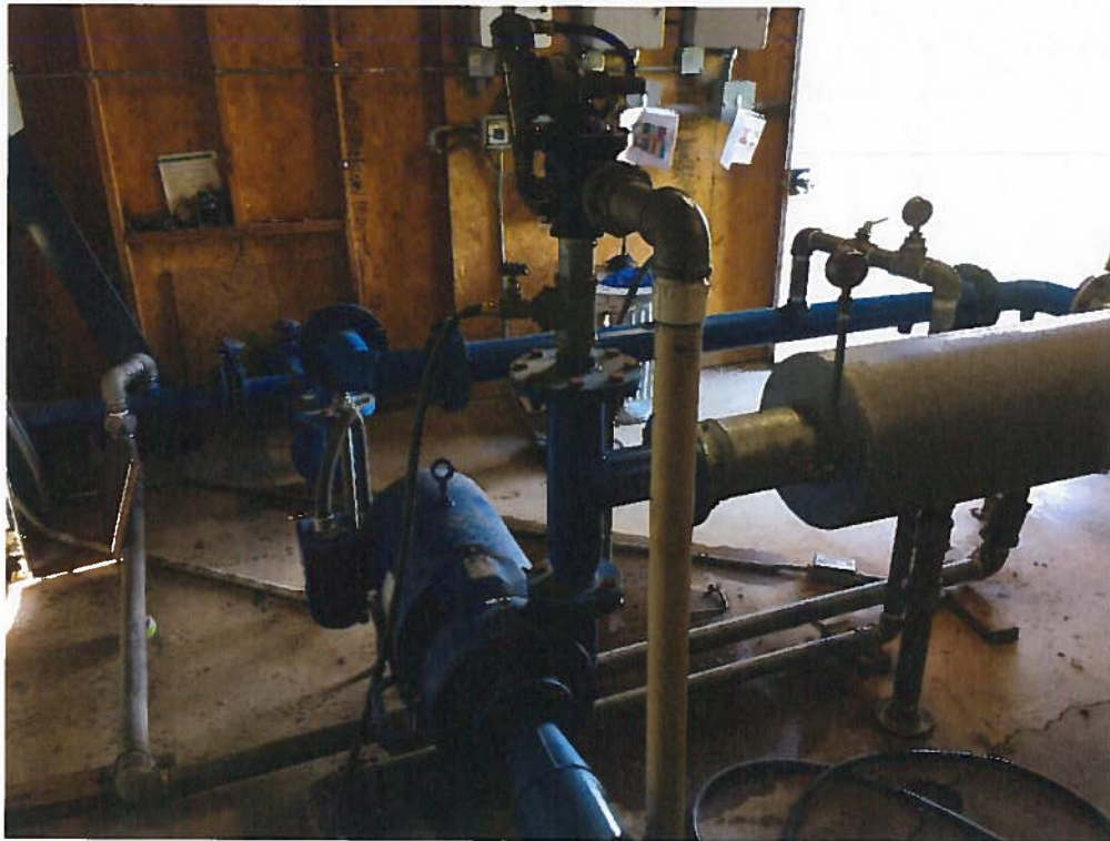
Surface water pump system for pond 2
