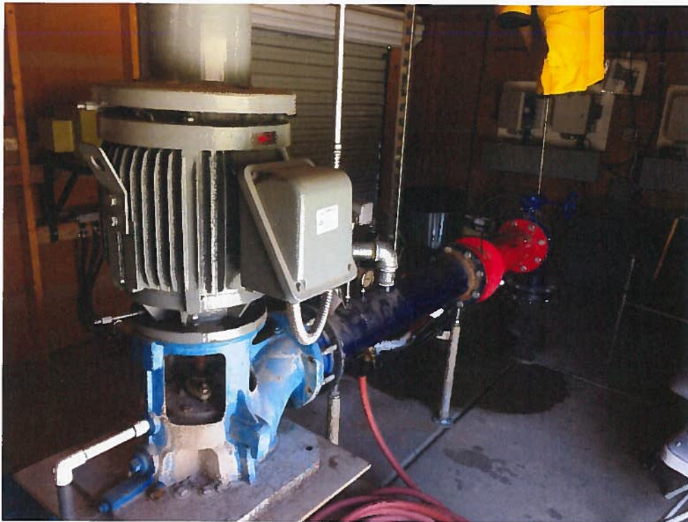
Surface water pump system for pond 1
