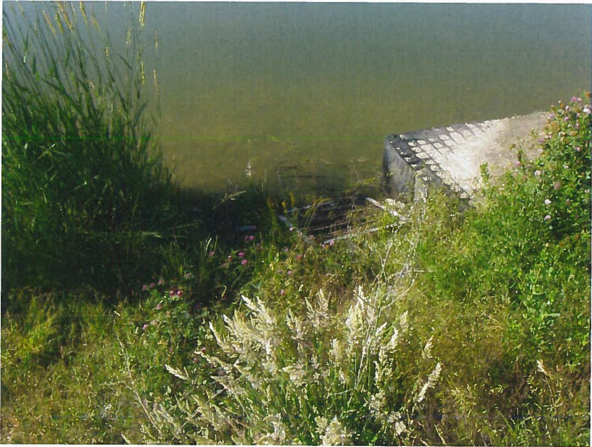
Overflow outlet on north side of pond 1
