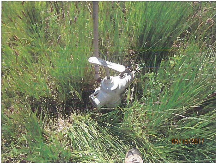
Figure 6 The risers which tie into wheel lines for irrigation.
