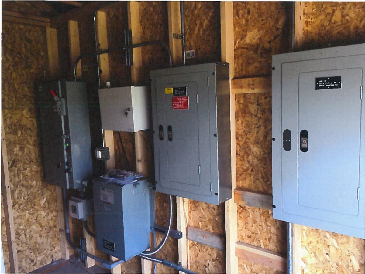
Electrical panels in irrigation pump station. Well pump panel on far left. Well pump starts and stops based on pond level using level sensors.
