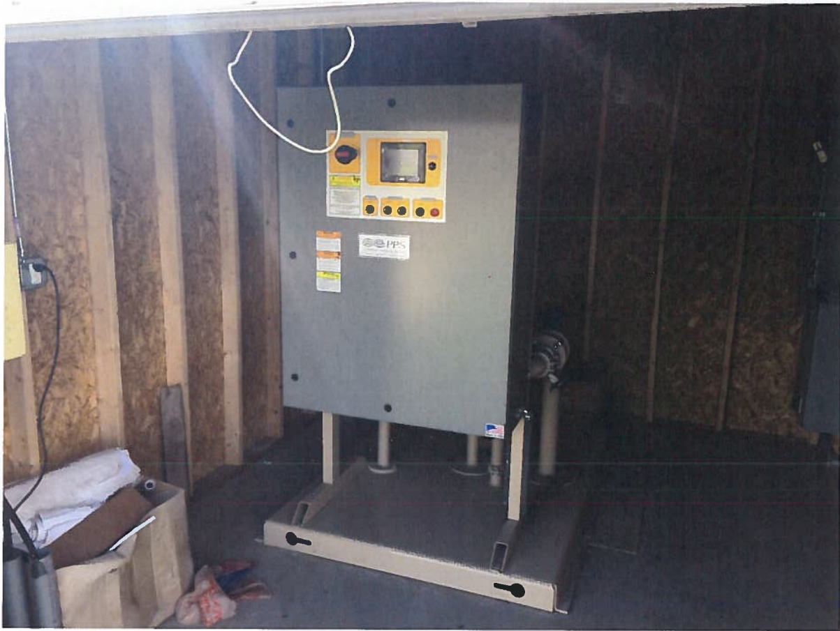
Control panel on irrigation pump skid. Submersible pumps for pressure irrigation system are in wet well below the pump skid.
