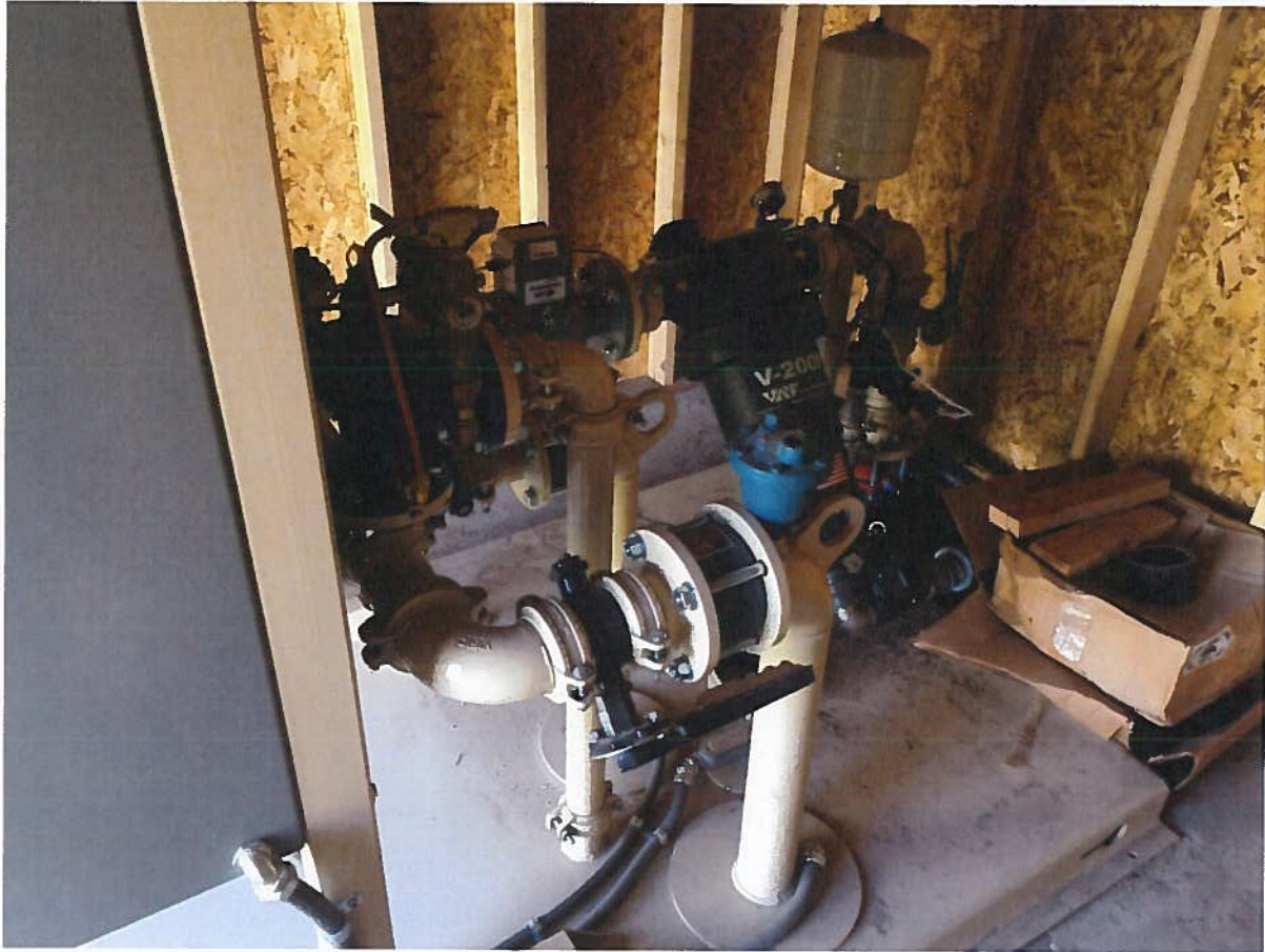
Discharge valves and mechanical equipment on pump skid.
