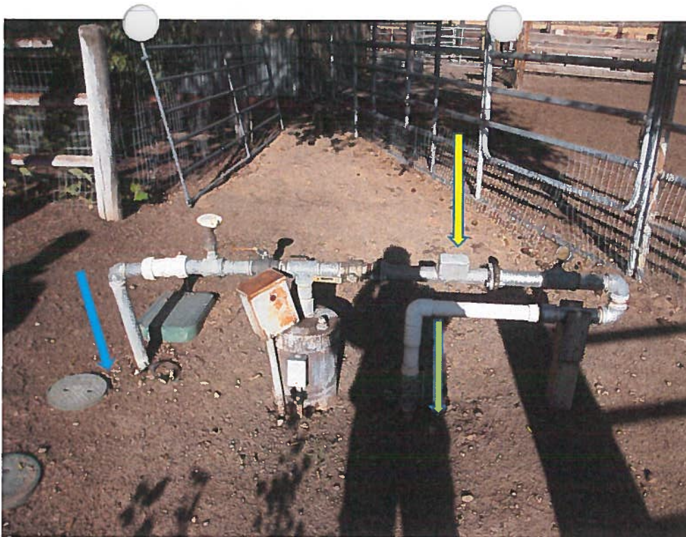
Well head and piping to domestic use (blue arrow) and irrigation use (green arrow). Flow meter is at yellow arrow.
