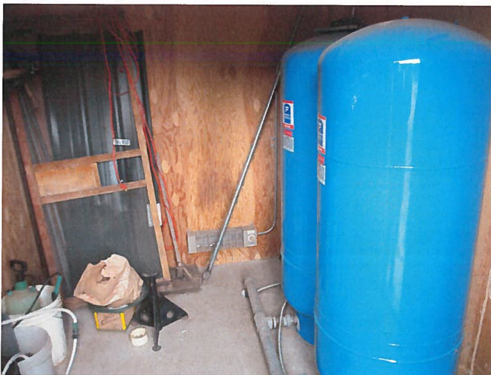
Plumbing inside pump house
