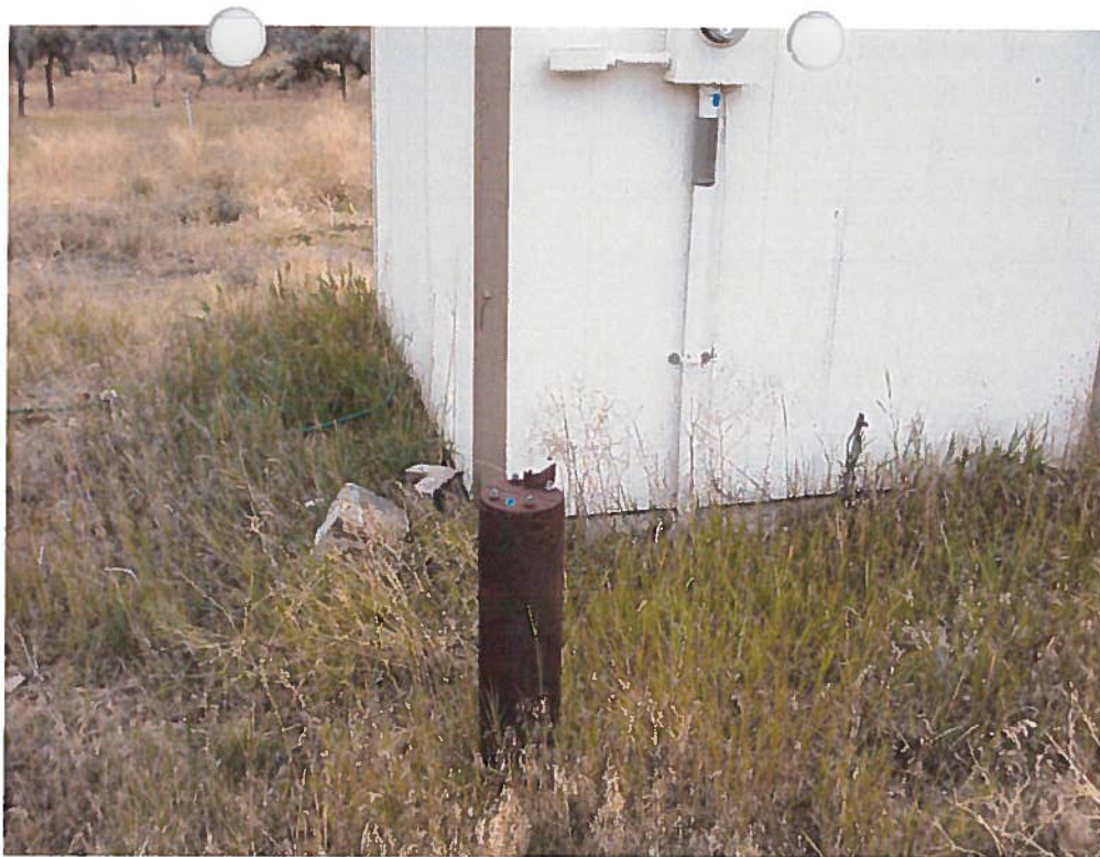
Well head near pump house
