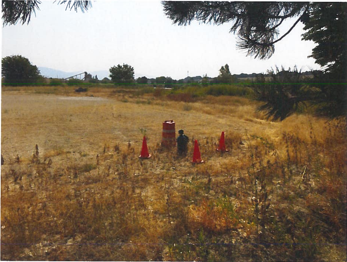
Point of Diversion: 8-inch well and submersible pump in SESW Section 22. Pump discharges through a pitless connection to 6-inch buried pipeline approximately 500 feet to Watershed exhibit.
