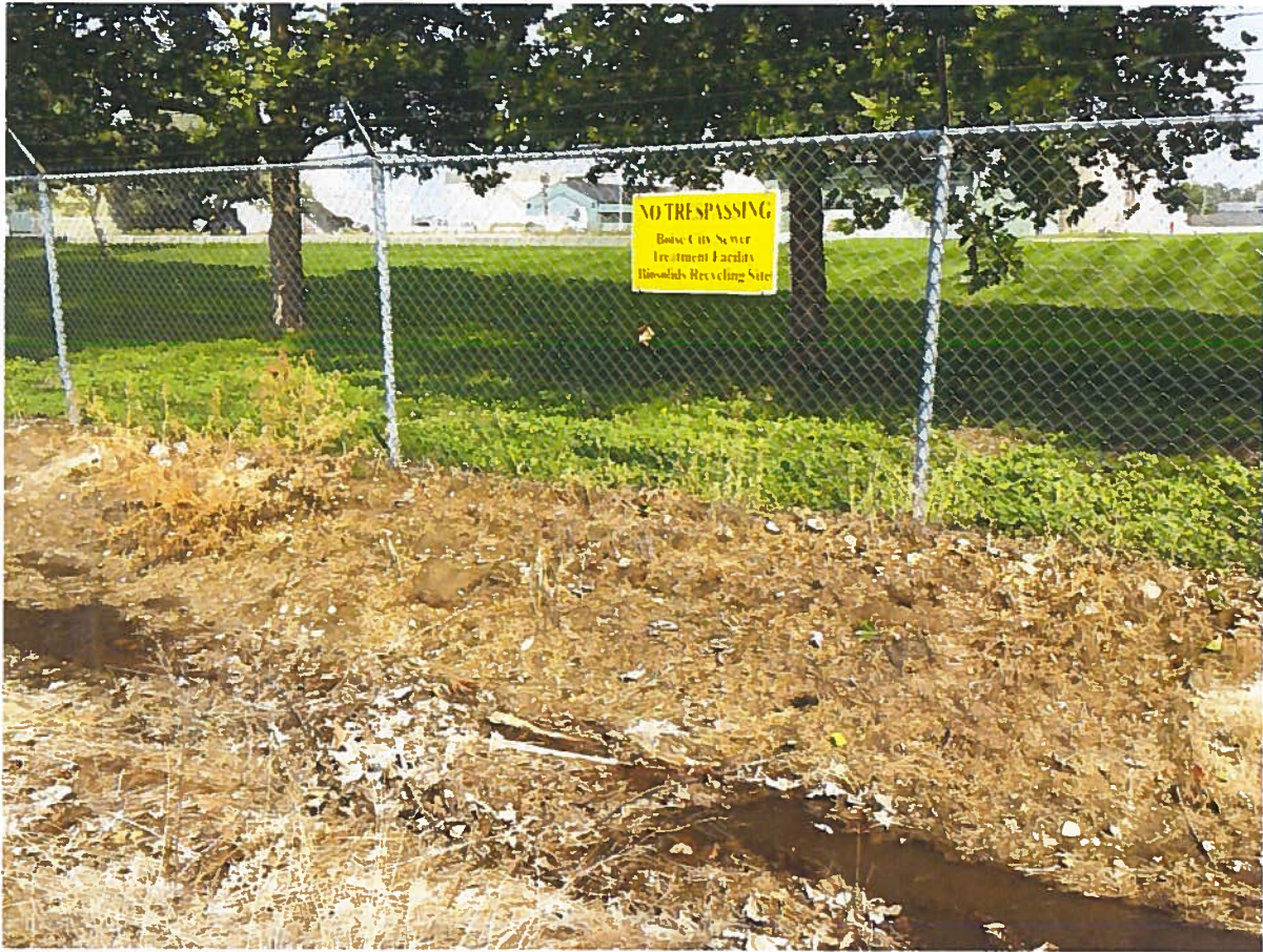
Water infiltrating in open ditch on south side of wastewater treatment plant fence
