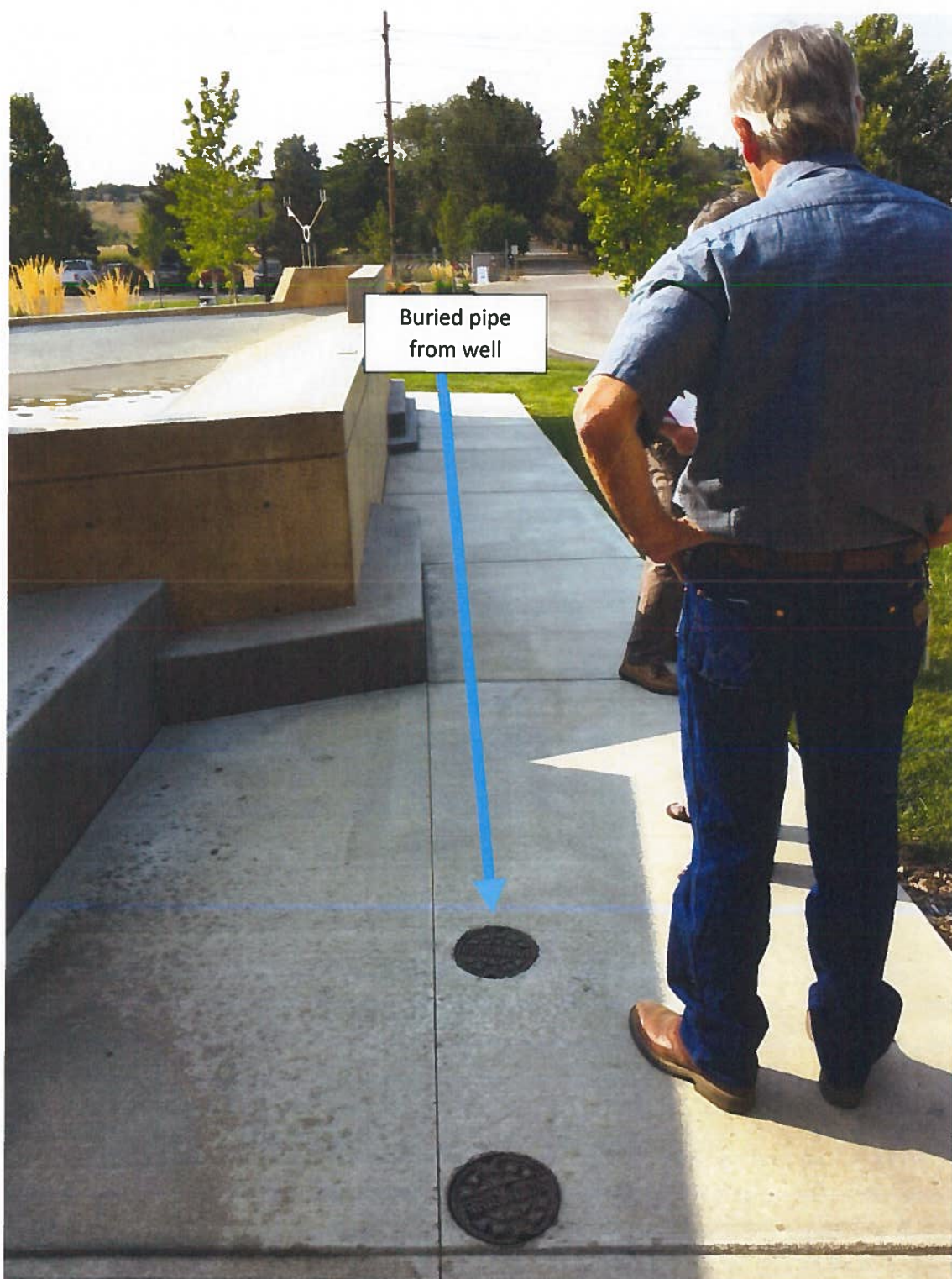
Upper valve cover is for isolation valve between well and storage reservoir and fountain. Lower valve cover is for drain to treatment plant for fountain flows during winter months.
