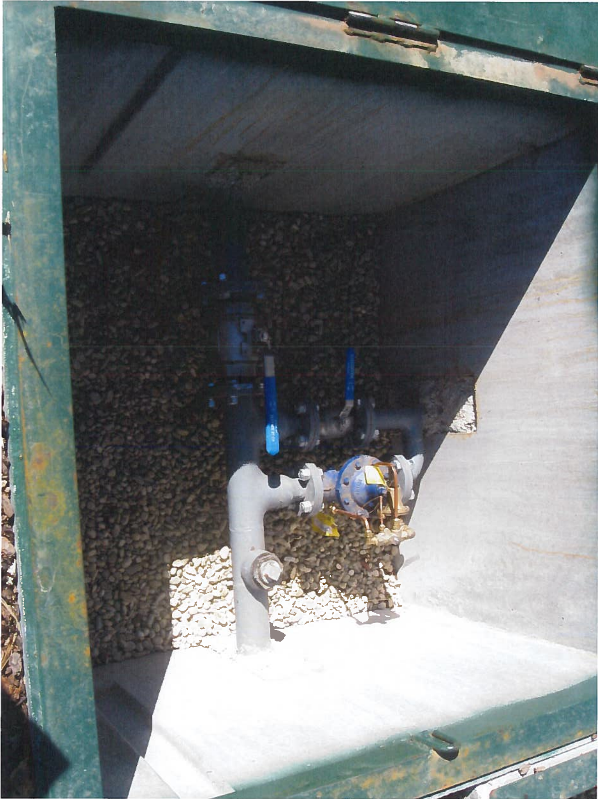
Vault with isolation valve, flush to waste valve, and pressure relief valve.
