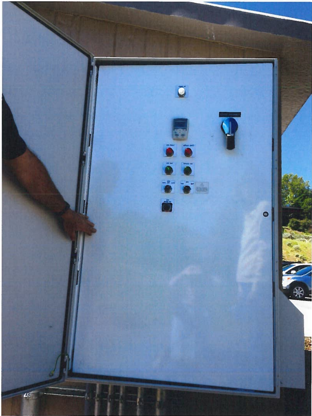
Door of pump control panel.
