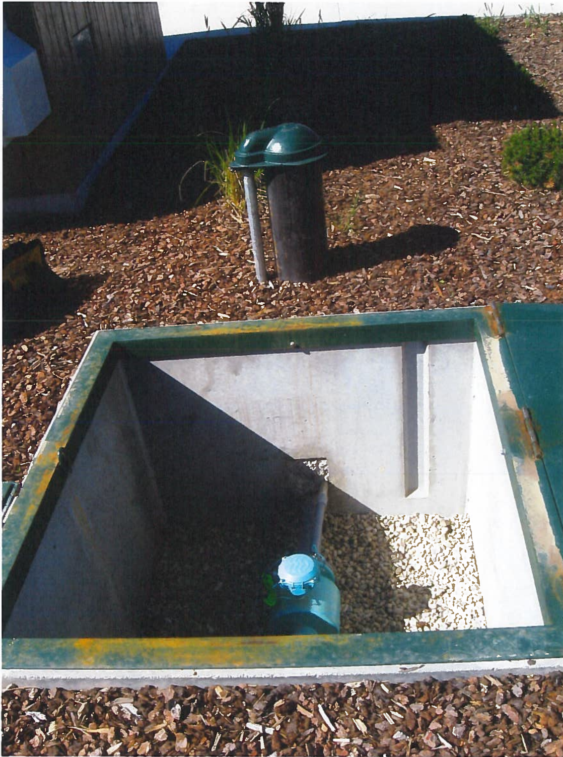
Irrigation well head with adjacent vault containing flow meter and pressure transducer. Submersible well pump discharges through a pitless adapter to the vault.
