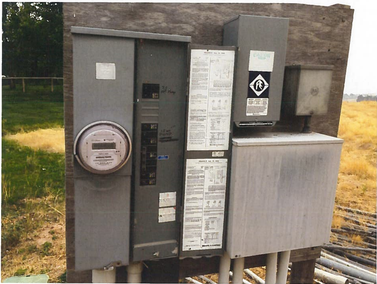
Pump electrical controls
