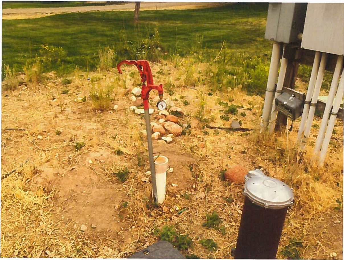
8-inch well and yard hydrant for pressure measurement.
