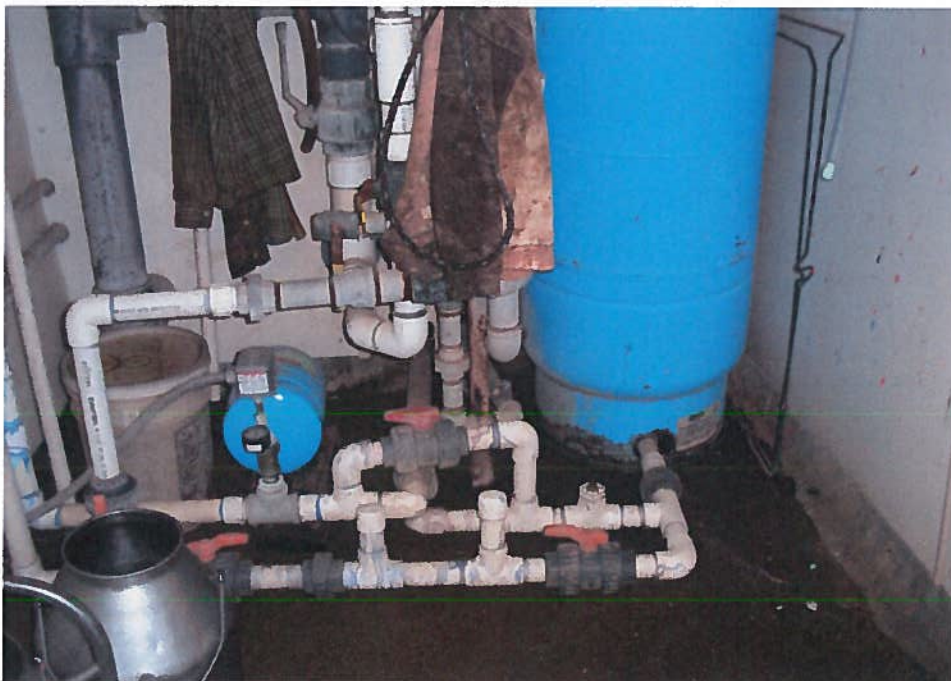
Figure 2 Plumbing leading into the pressure tank from the well.
