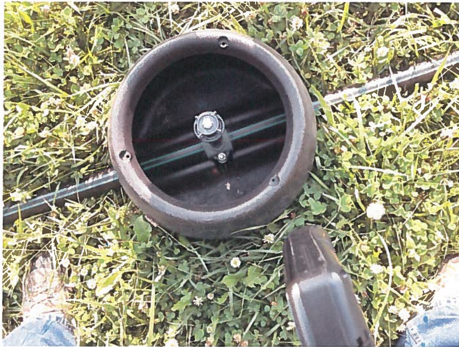
Figure 5 There are 23 sprinkler heads distributed amongst 5 sprinkler pods. Each sprinkler is rated for 4.7 gpm at 65 psi pressure.
