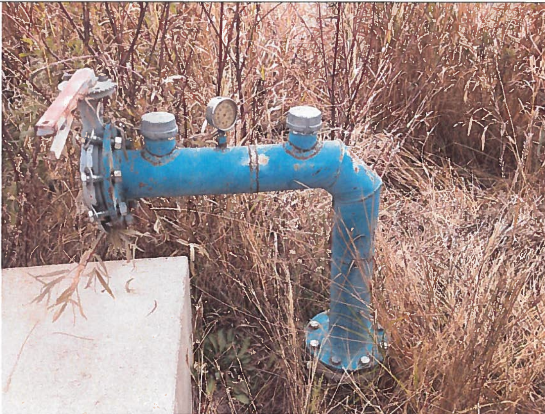
Main line for Pump System#2
